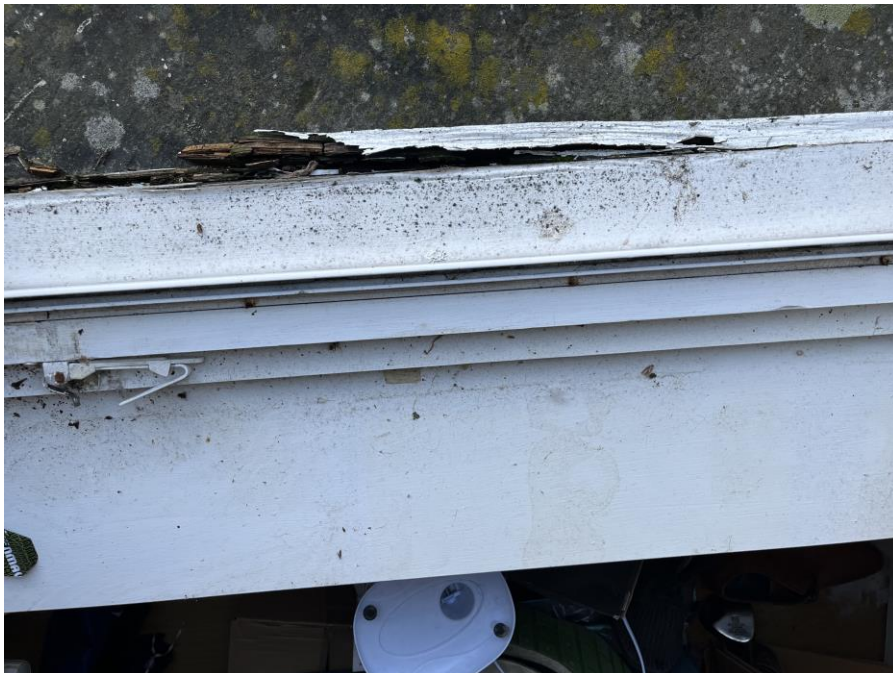
Rotten window sill
