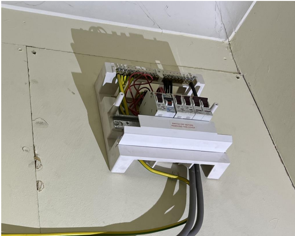
Missing cover on the electricity consumer unit
