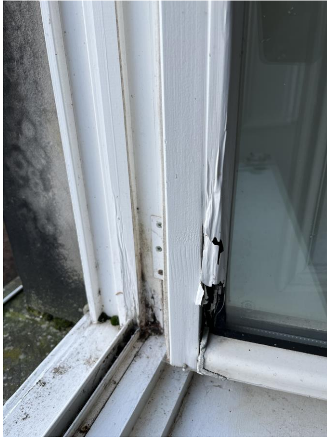
Rotten window frame
