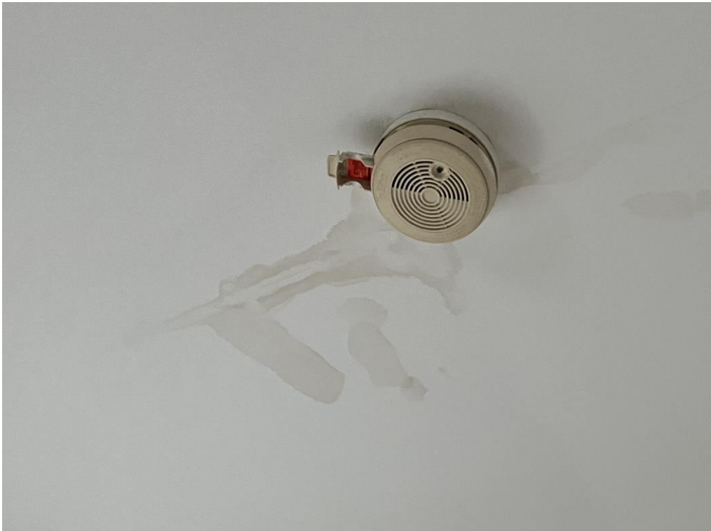
Stain marks on the ceiling and battery powered smoke detector
