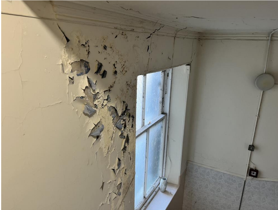
Historic damp penetration on the common stair
