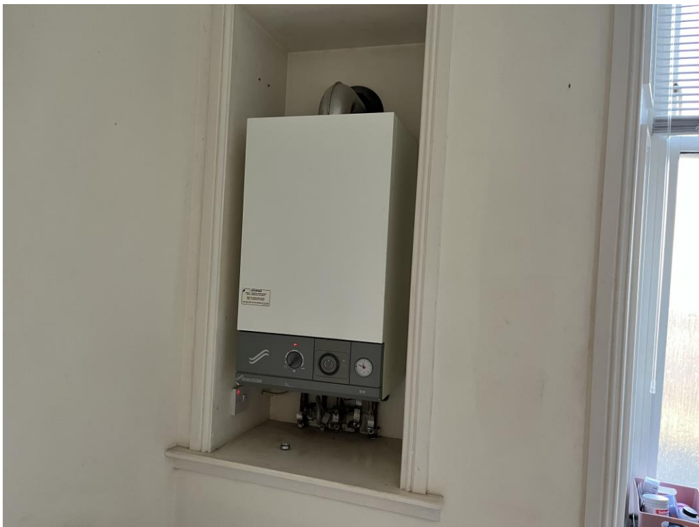
Gas fired boiler in the bathroom
