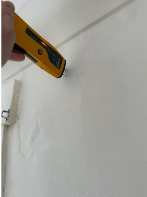
Photograph 6: Bedroom 1: damp meter reading adjacent window head (high levels of moisture present)
