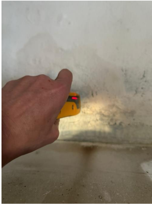
Photograph 4: Bedroom 1: damp meter reading to upper inside of wardrobes (high levels of moisture present)
