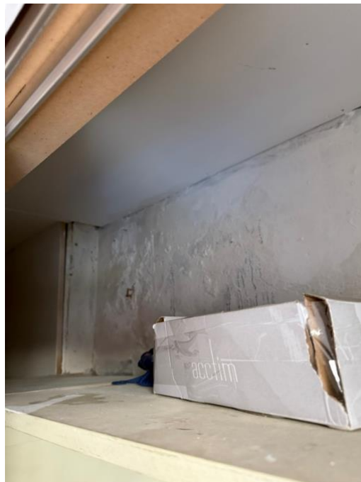
Photograph 3: Bedroom 1: to upper inside of wardrobes
