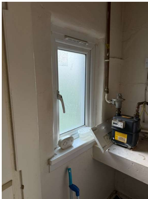
Photograph 3: Carbon monoxide detector on boiler room windowsill
