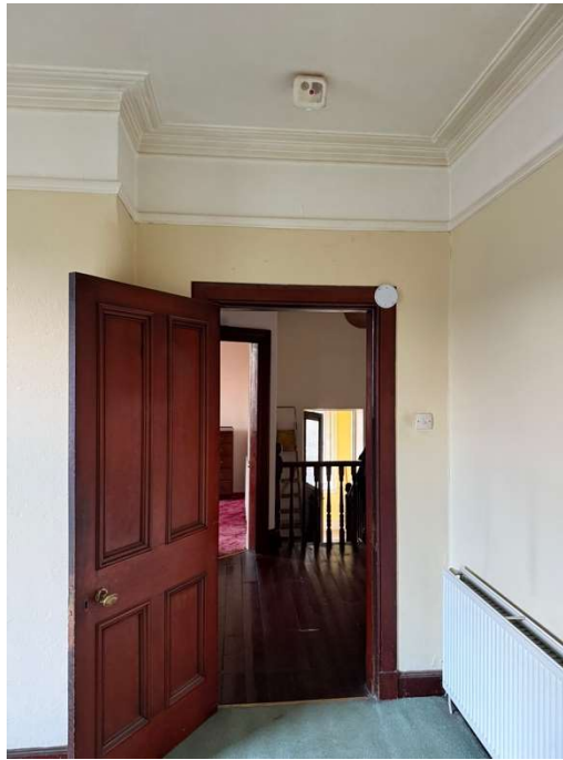
Photograph 6: Living room – no working smoke detector
