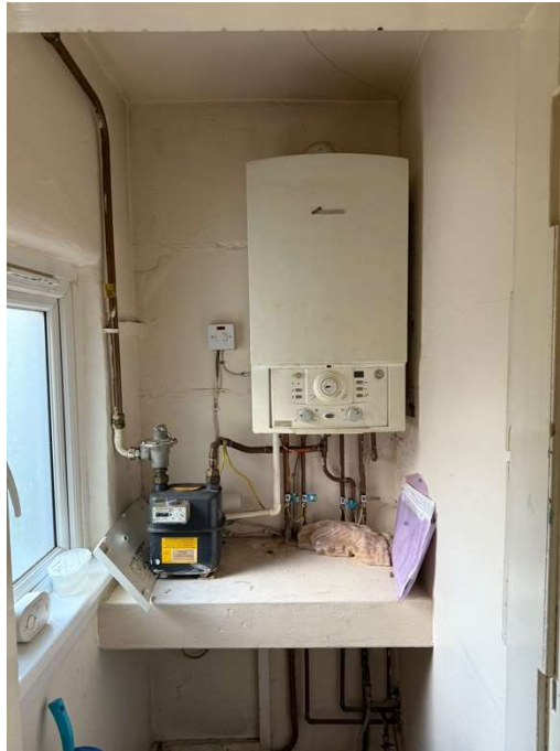
Photograph 2: Gas boiler – in room off kitchen
