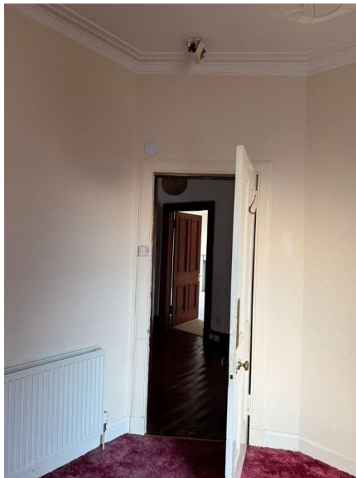
Photograph 7: Bedroom 1 – no working smoke detector
