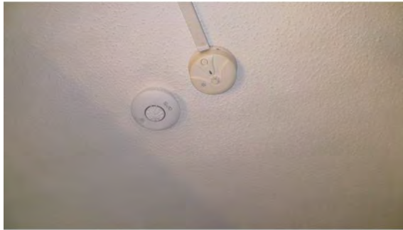
Photo 12 – Smoke detector in Hallway
