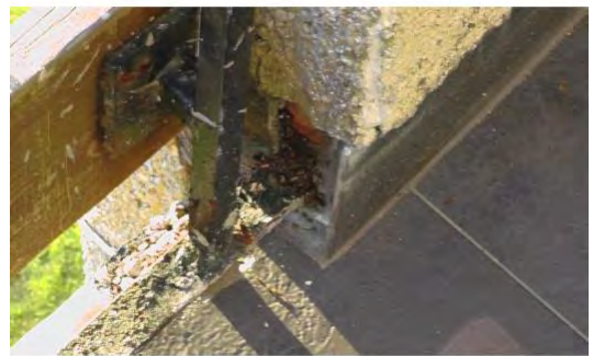
Photo 5 – Unfinished Balcony wall/edge repair
