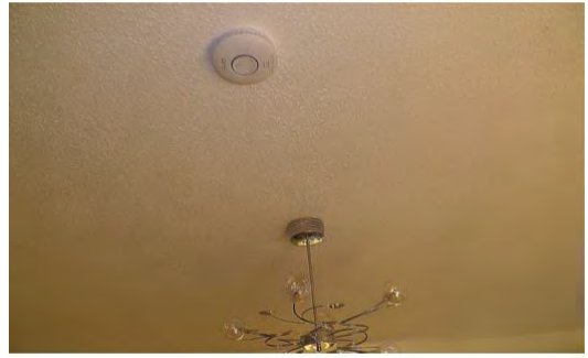
Photo 11 – Smoke detector in Living Room
