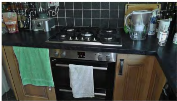
Photo 14 – Faulty cooker unit
