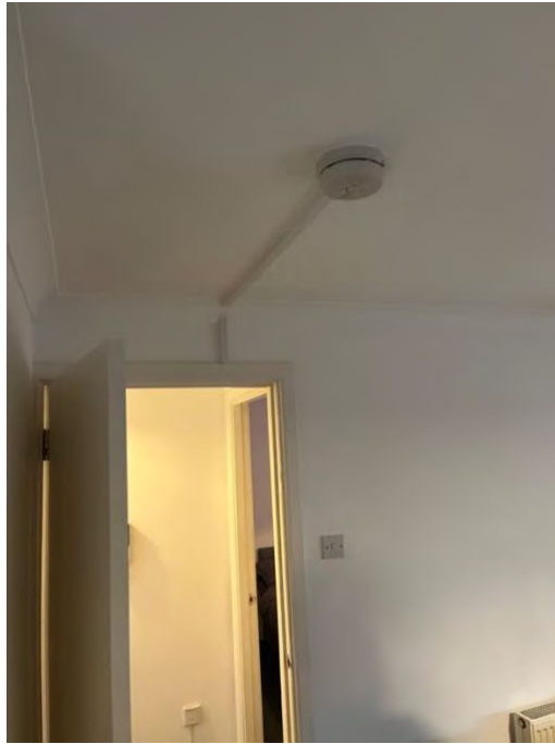
Photograph 6: Living room – smoke detector
