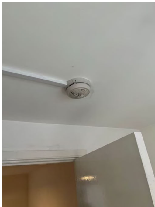
Photograph 5: Kitchen – heat detector
