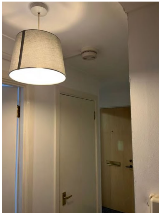
Photograph 7: Hallway – smoke detector
