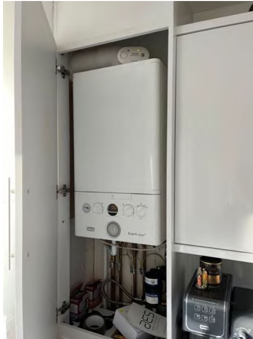
Photograph 2: Gas boiler – kitchen cupboard with carbon monoxide detector
