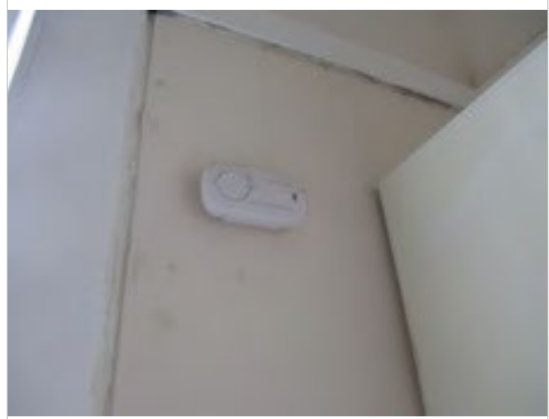
Kitchen - wall mounted carbon monoxide detector - does not appear to be in working order/position does not comply with guidance (observation)
