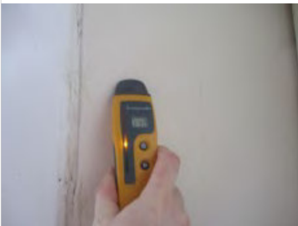
Kitchen - plasterboard panel to right side of window - damp meter reading - moderate in search mode
