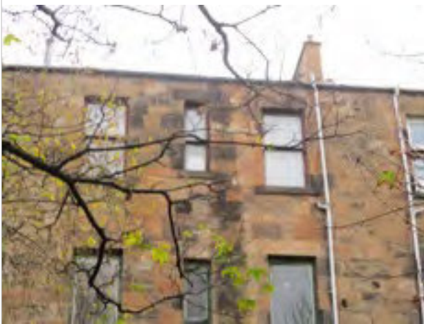
External - rear elevation showing rainwater and waste pipes - staining to stonework below gutter and extending towards ground level
