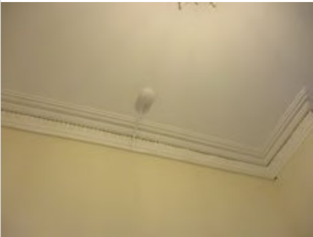
Hall - ceiling mounted smoke detector - tested and in working order/interlinked (observation)
