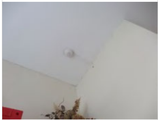
Kitchen - ceiling mounted heat detector - tested and in working order/interlinked (observation)
