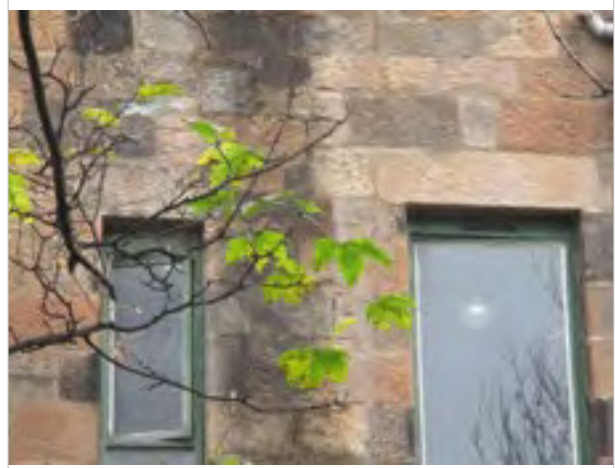
External - rear elevation showing kitchen and bathroom windows - extensive water staining to stonework from gutter above and between window openings
