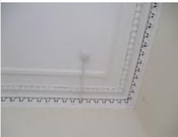
Living Room - ceiling mounted smoke detector - tested and in working order/interlinked (observation)
