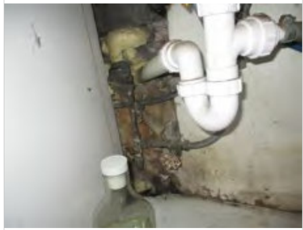
Kitchen - below sink at rear elevation - large gap/ exposed stonework to rear of base unit
