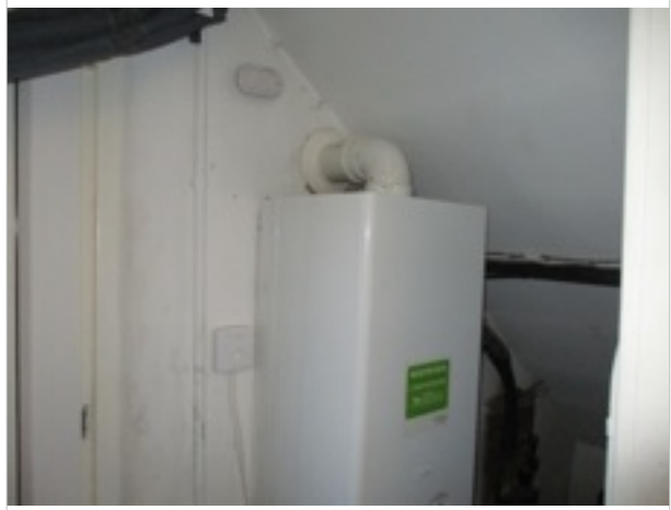
Hall - boiler and carbon monoxide detector
