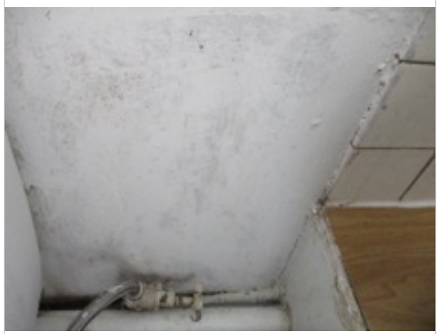
Bathroom - rear external wall - moisture build up on wall surface
