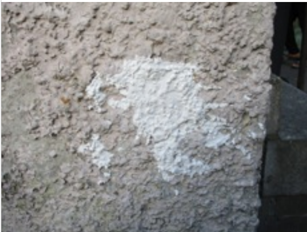
Rear Elevation - roughcast patched
