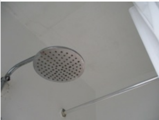
Bathroom - ceiling above bath
