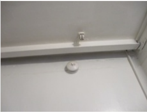
Kitchen - wall mounted heat detector (observation)
