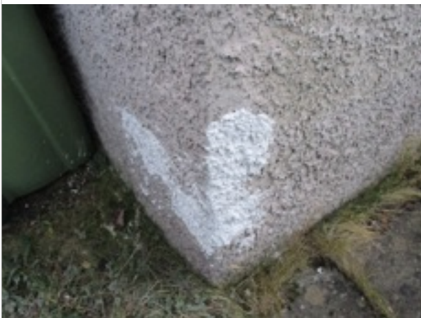
Corner of Hip End and Front Elevation - roughcast patched
