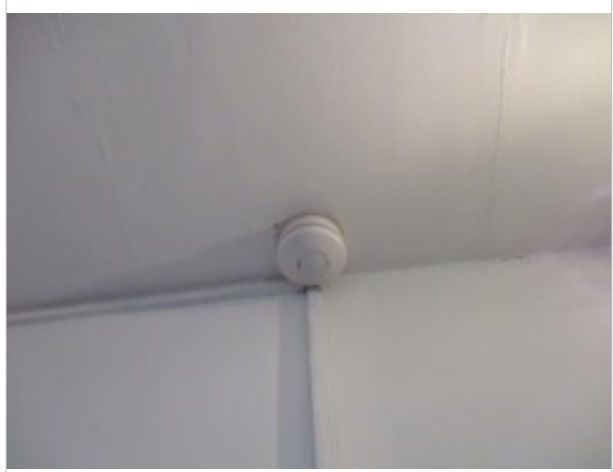
Hall - ceiling mounted smoke detector (observation)
