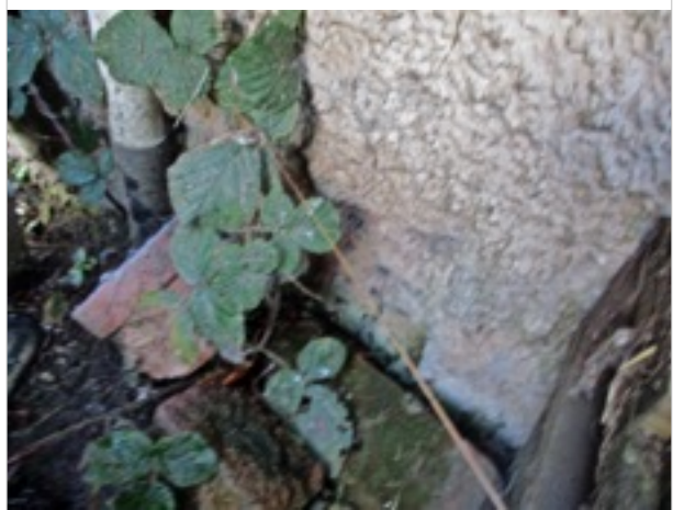
Rear Elevation - underfloor vent to left of back door - part obscured by ground level
