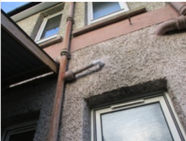
Rear Elevation - cast iron downpipe and repaired waste pipe from UF flat
