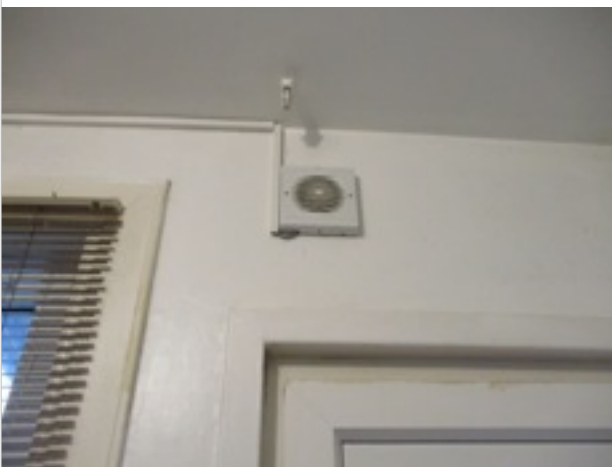
Kitchen - extractor fan
