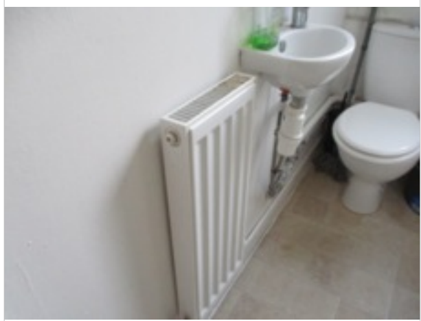
Bathroom - new radiator
