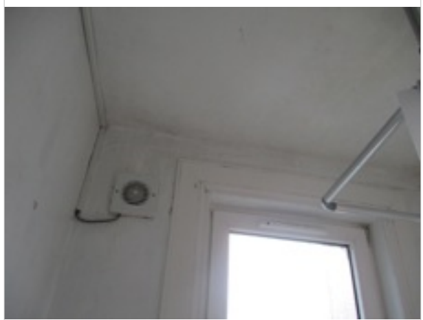
Bathroom - extractor fan
