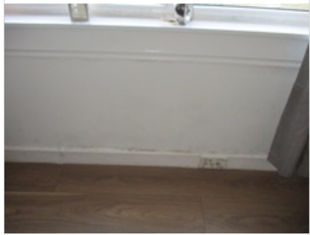
Living Room - front external wall below window
