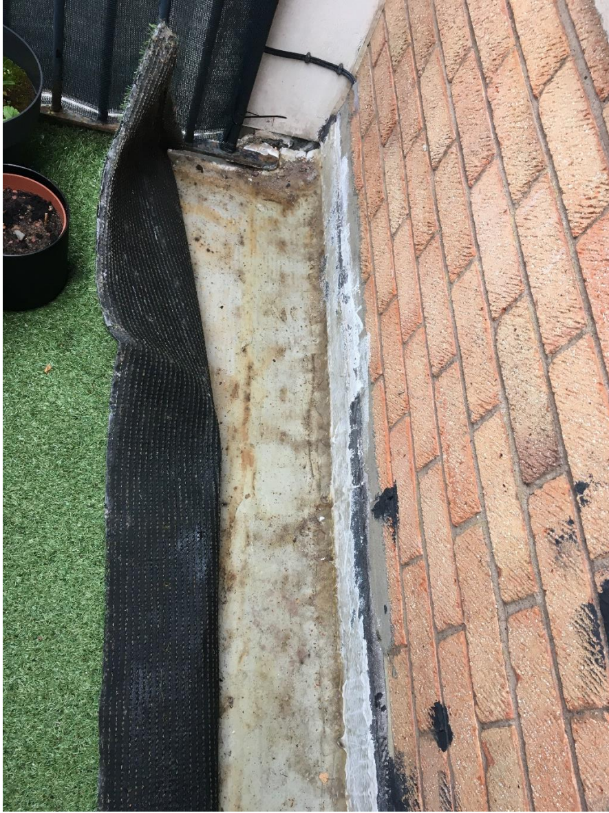
The flashing at the foot of the exterior wall of the balcony has not been replaced satisfactorily.
