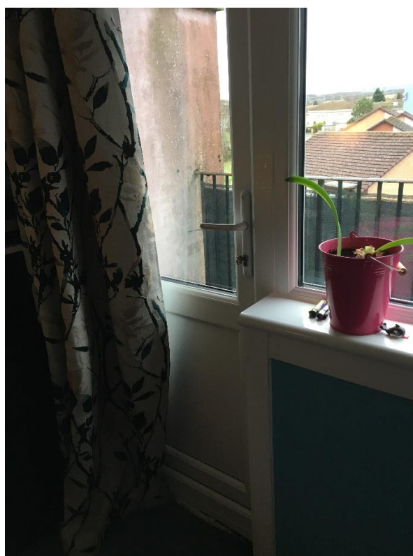
The door and door frame leading from the living room to the balcony have been replaced.
