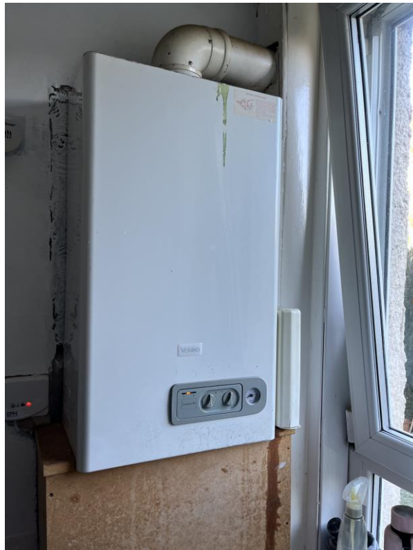
Gas fired boiler
