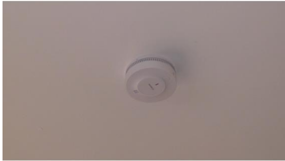
Photo 10 – Functioning smoke detector in Living Room
