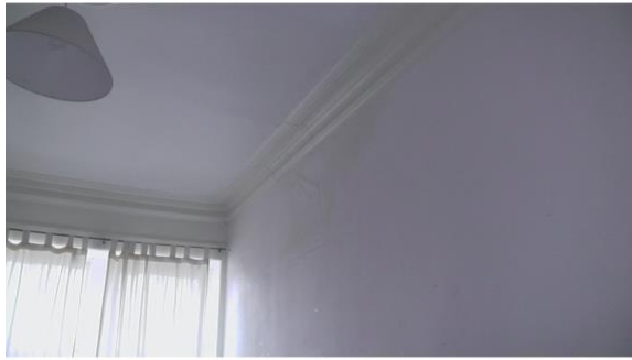
Photo 2 – Damp free Bedroom wall + historic water ingress staining
