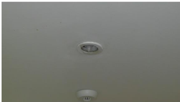
Photo 8 – Functioning heat detector in Kitchen
