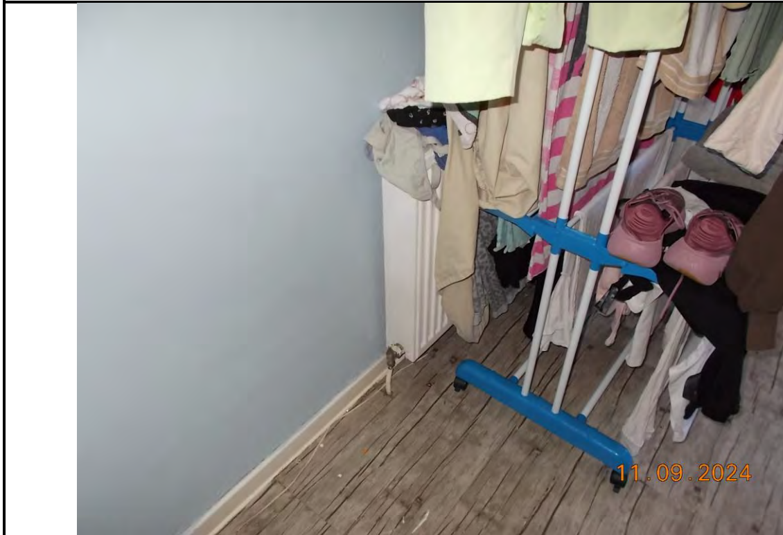
3. Living Room Radiator
