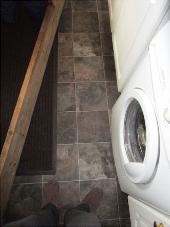
9. Hazardous floor in kitchen
