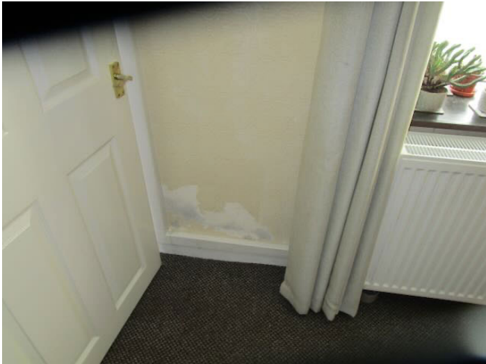
1. Damp patch in Living Room.
