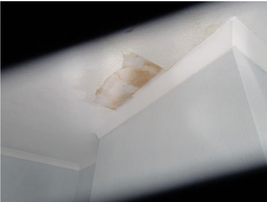
8. Damp patch at ceiling adjacent chimney breast in bedroom.
