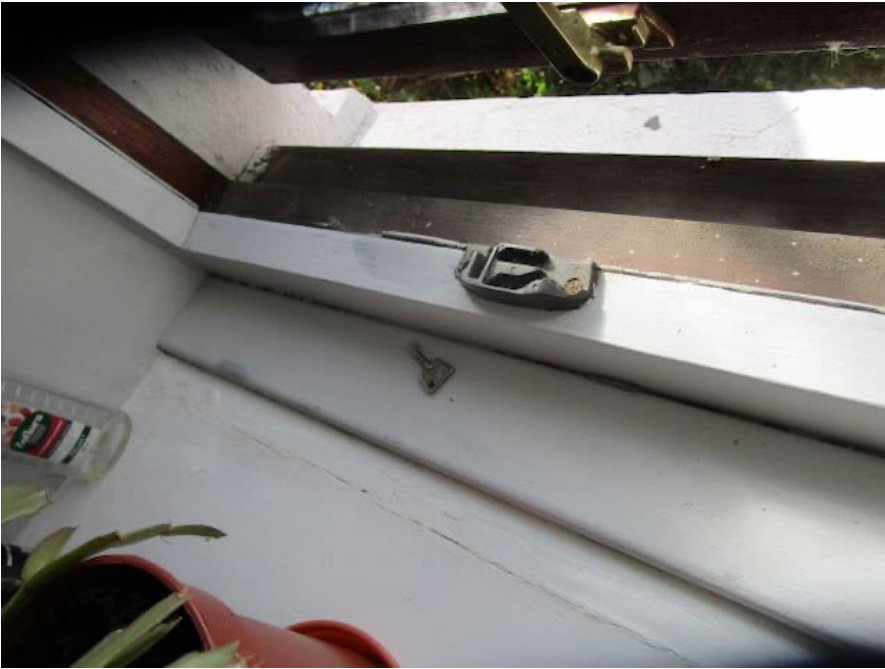
7. Damaged seals at bathroom window
