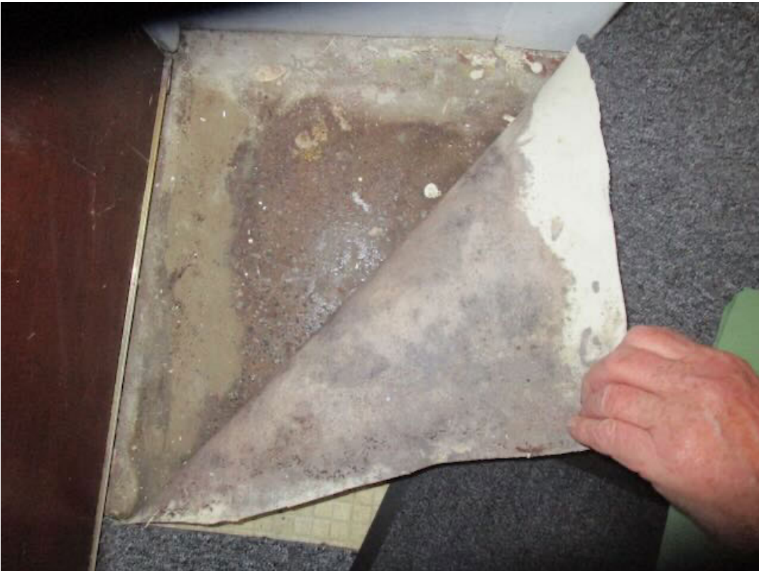
6. Damp concrete floor adjacent front door.
