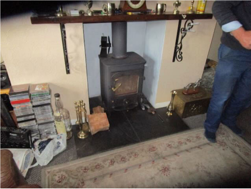
3. Multi fuel burner and flue.
