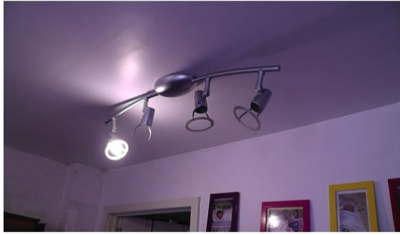
Photo 26 – Broken light fitting in Utility room
