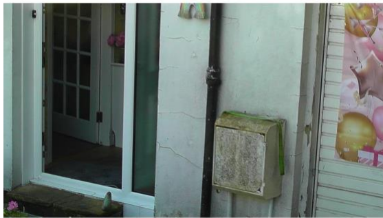
Photo 22 – Cracking on render
