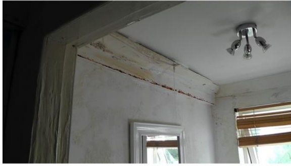
Photo 2 – Water damage in WC
