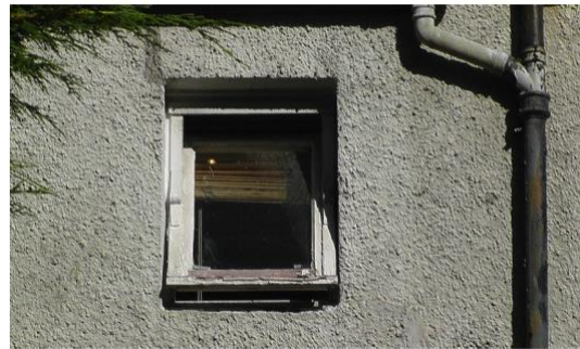
Photo 25 – WC window issues
