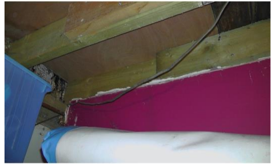
Photo 11 – Continuation of loose cable
