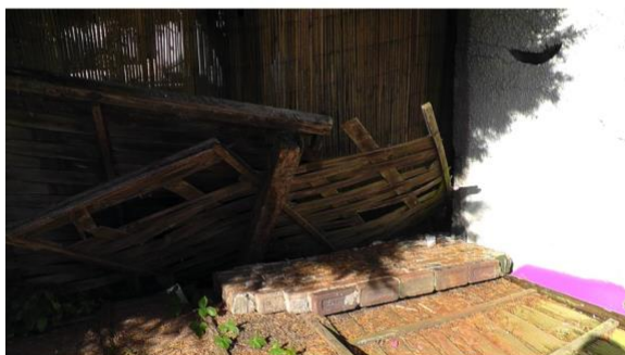
Photo 16 – Collapsed fence panels and wall section
