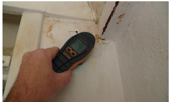
Photo 7 – Embedded dampness reading in WC
