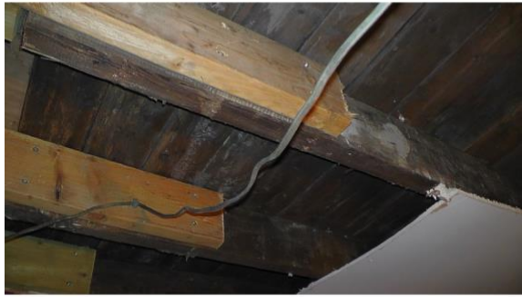
Photo 10 – Loose electrical cable in garage
