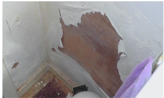
Photo 5 – Water damage in WC
