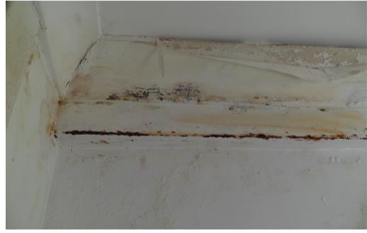
Photo 3 – Water damage in WC
