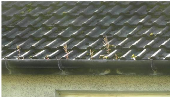
Photo 12 – Choked gutter on front elevation
