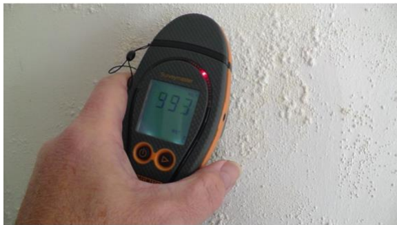
Photo 6 – Embedded dampness reading in WC
