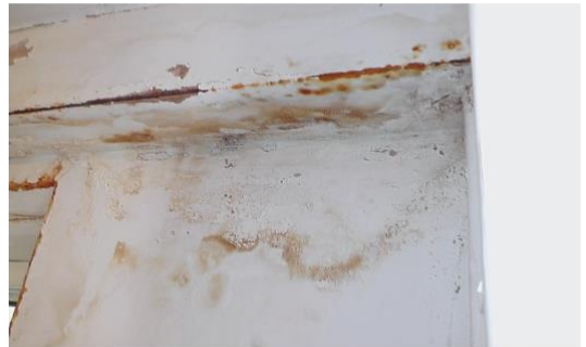
Photo 9 – Water damage in Utility room
