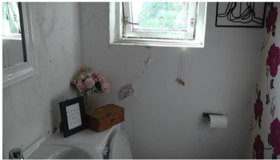
Photo 4 – Water damage in WC
