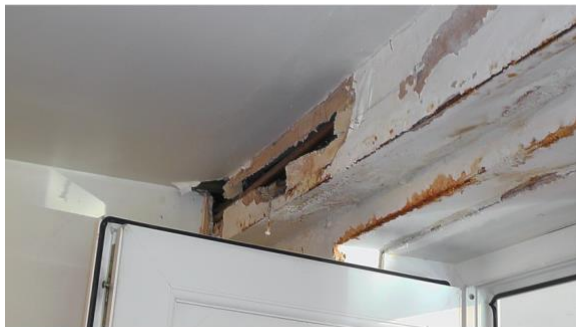
Photo 8 – Water damage in Utility room
