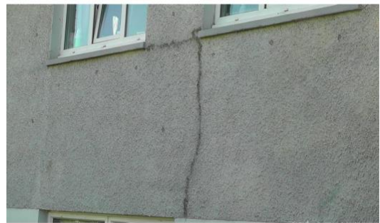
Photo 23 – Roughcast issues on front elevation
