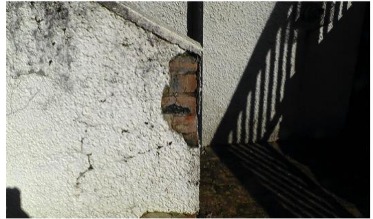
Photo 21 – Roughcast issues/exposed brickwork
