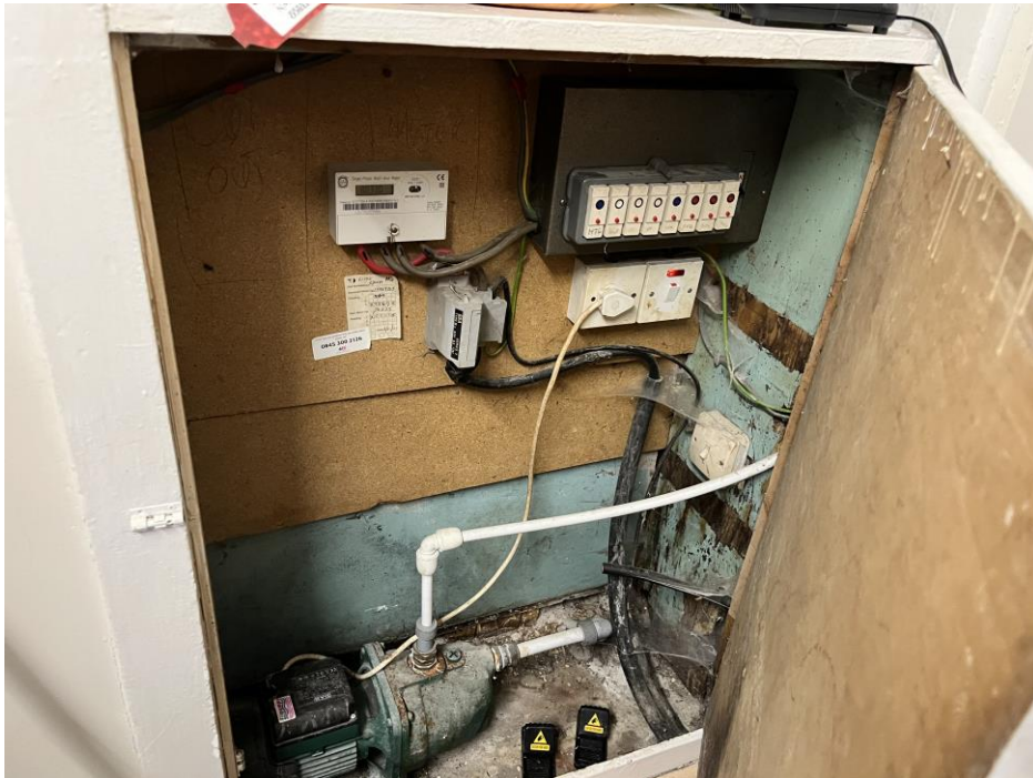
Electrical consumer unit
