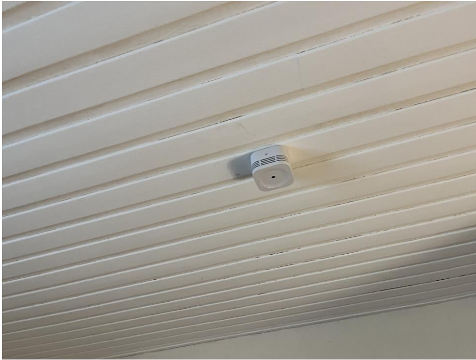
Smoke detector in the Living-room
