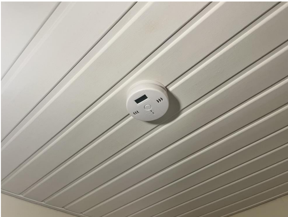
Carbon monoxide detector in the hall
