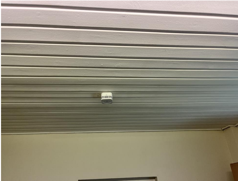
Smoke detector in the kitchen
