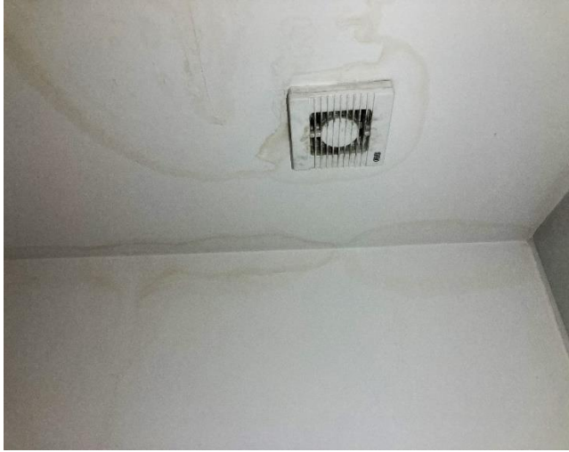
27 February 2024 - Bathroom vent
