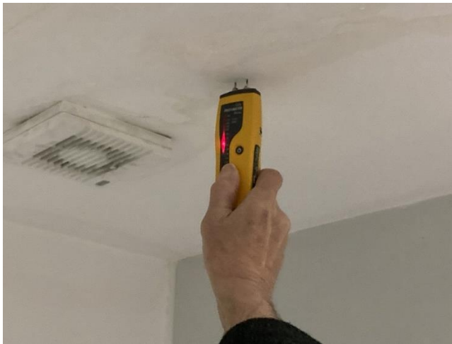
27 February 2024 – Damp readings
