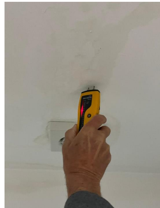
30 August 2024 – Damp readings
