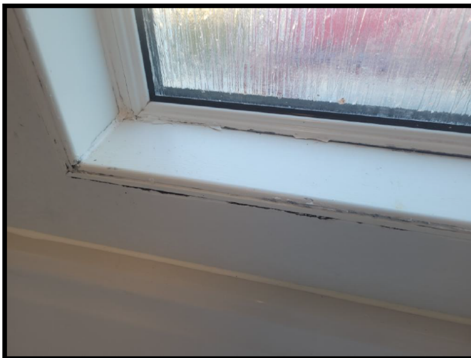
Photograph 5 Bathroom: Mould to silicon sealant.
