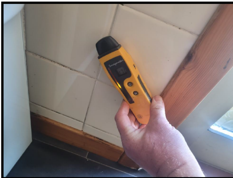
Photograph 7 Kitchen: Moisture meter reading 17% near cooker and outer door.
