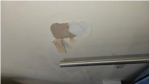
11 Towel rail support bracket secured by adhesive pad which has failed within Bathroom.
