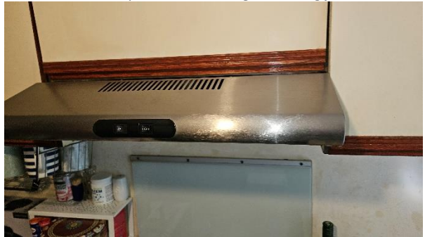
4 Cooker hood – recently replaced.
