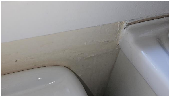
13 Minor imperfections evident to decoration in Bathroom.
