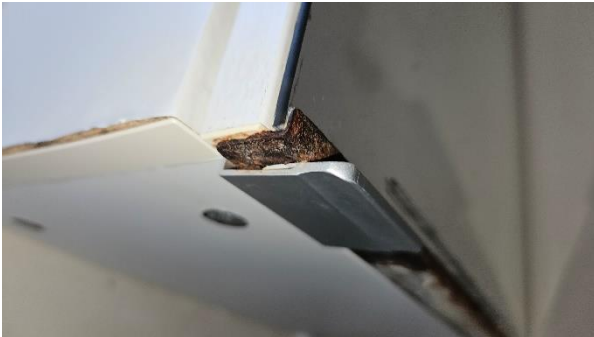
9 Bathroom cabinet - "L" shaped metal retention trim corroded.
