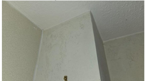
12 Bathroom walls – minor mould growth evident to external wall.
