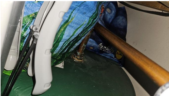
15 Hot water cylinder.
