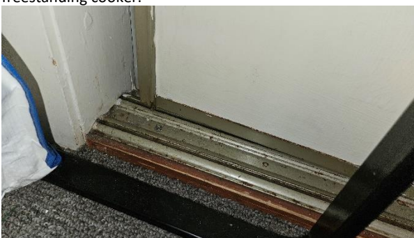
7 Bottom of door disengaged from sliding track (bedroom wardrobe).
