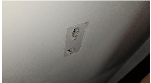
10 Bathroom walls – redundant fixing holes evident from previous fixtures/fixings.
