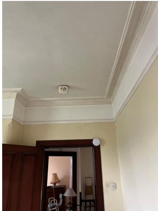
Photograph 6: Living room – smoke detector to door frame
