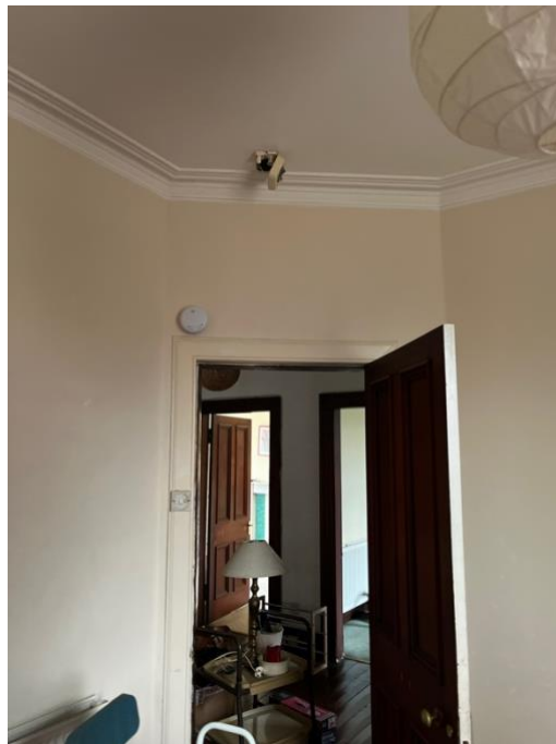
Photograph 7: Bedroom 1 – smoke detector just above door frame
