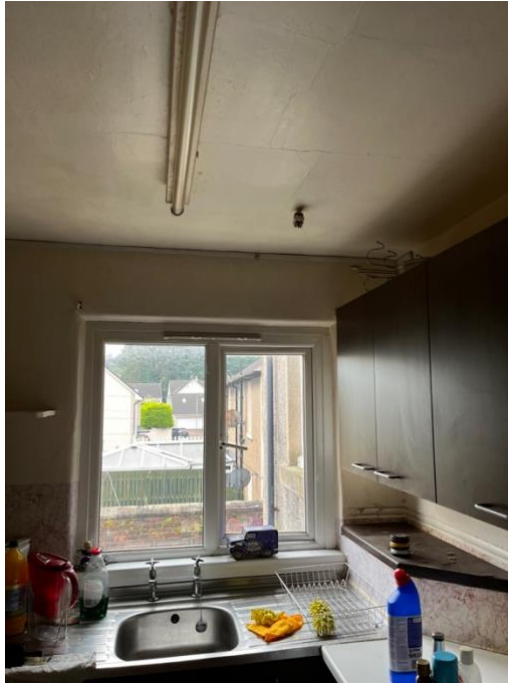
Photograph 4: General view of kitchen – no heat detector to ceiling
