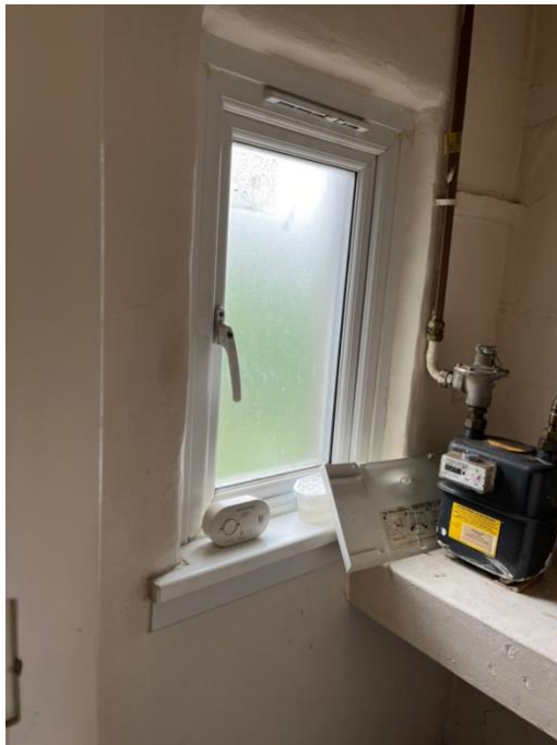
Photograph 3: Carbon monoxide detector on boiler room windowsill
