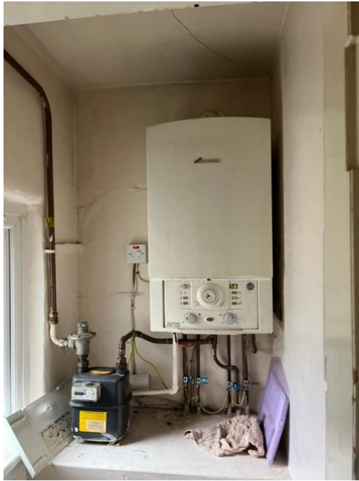
Photograph 2: Gas boiler – in room off kitchen
