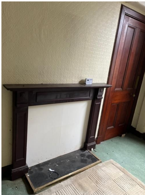
Photograph 5: Living room - carbon monoxide detector on fireplace
