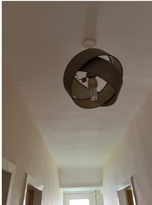
Photograph 4: Hallway ceiling: no smoke detector
