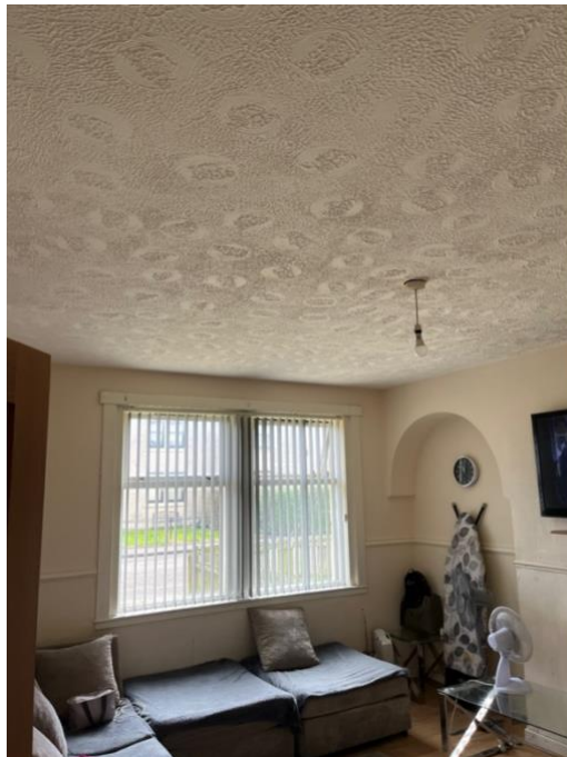
Photograph 3: Living room: no smoke detector
