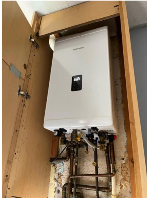
Photograph 2: Kitchen: gas boiler – no carbon monoxide detector
