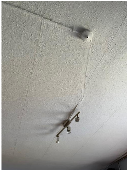
Photograph 5: Kitchen ceiling: no heat detector
