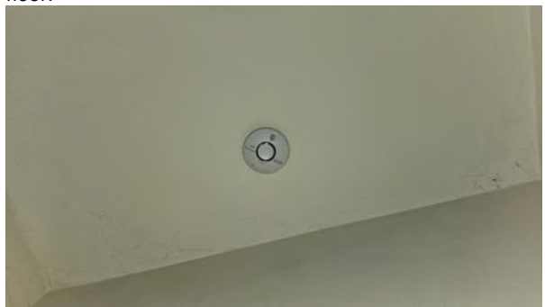
24 Smoke detector (not tested).
