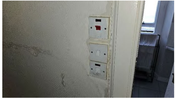
10 Water damage from adjacent shower enclosure into Hall in sphere of influence of electrical fittings.
