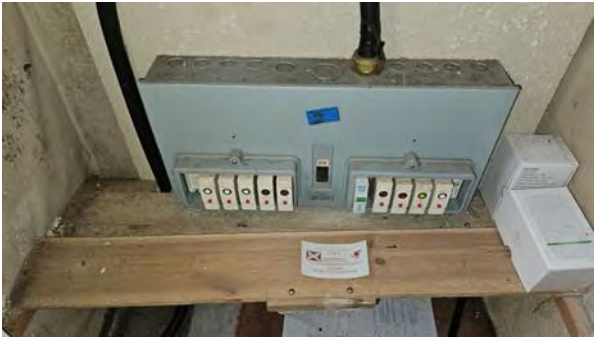
1 View of retrofit push-button MCBs to consumer unit.
