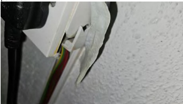
7 Damaged surface mounted backbox within Utility Room.
