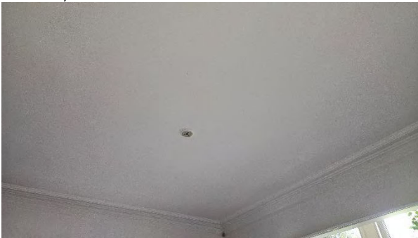
21 Redundant electrical fitting to ceiling.
