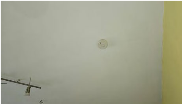
25 Detector in Kitchen (not tested).
