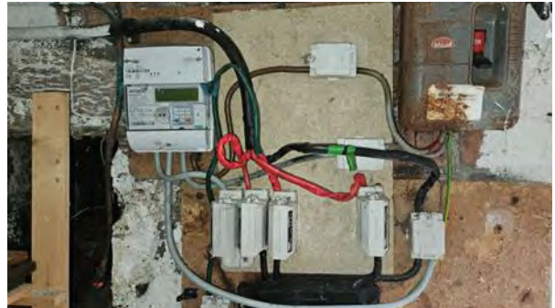
2 Incoming electrical supply, meter and switchgear.
