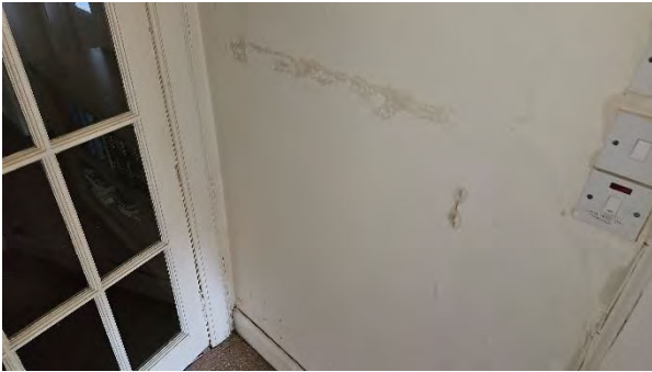
9 Water damage from adjacent shower enclosure into Hall in sphere of influence of electrical fittings.
