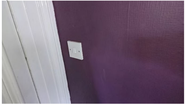
20 Example of redundant light switch
