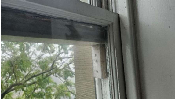
9 Timber blocks fitted to sash frame below top sash to prevent further slippage.
