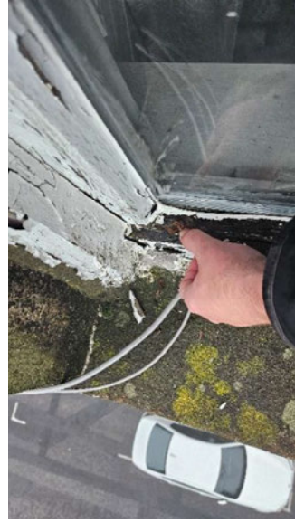
4 Living Room – south window (timber decay evident).
