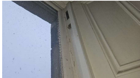
12 Rear Bedroom window – defective sash cords.
