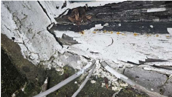
5 Living Room – south window (timber decay evident).
