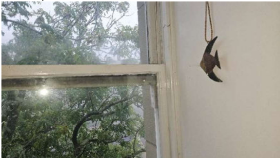
7 Kitchen window – misalignment of central rail due to top sash slippage.
