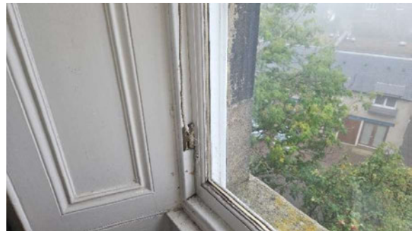
14 Rear Bedroom window – defective sash cords.
