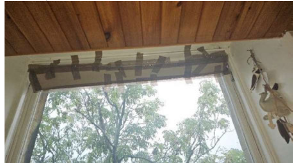
6 Kitchen window – temporary protection to gap above top sash unable to be closed.
