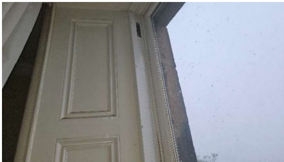
13 Rear Bedroom window – defective sash cords.
