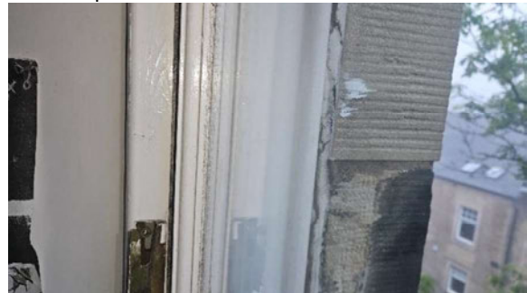
8 Defective perimeter sealant at Kitchen window.
