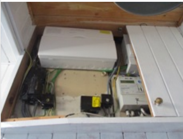
Ground floor front entrance vestibule - electric cupboard/consumer unit
