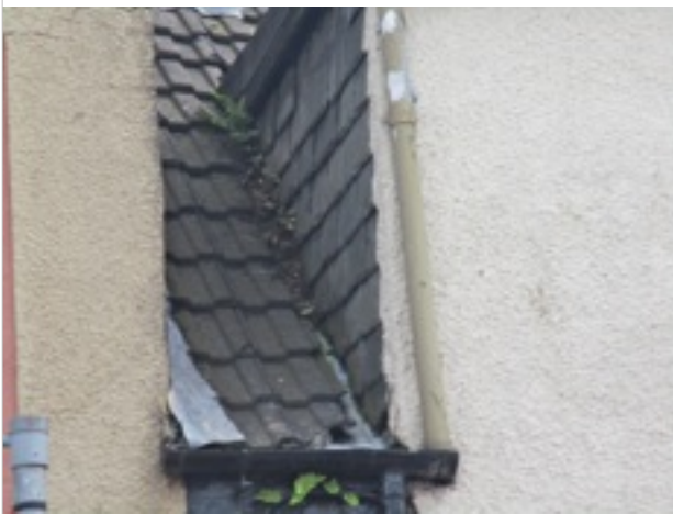
Front Elevation - vegetation growth on flashing at dormer and around gutter
