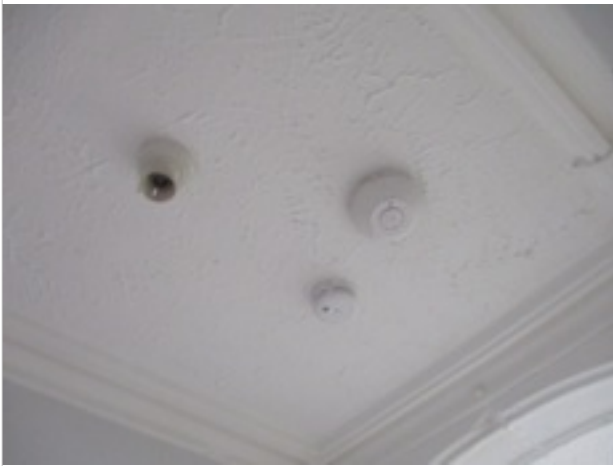
Ground Floor Hall - 2 x ceiling mounted smoke detectors
