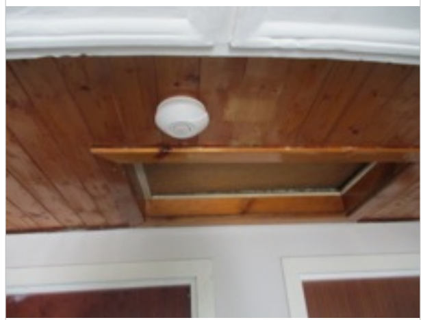
Upper Floor Landing - ceiling mounted smoke detector
