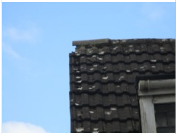
Rear Elevation - uneven tiles at roof verge and ridge/gap near ridge/broken tile
