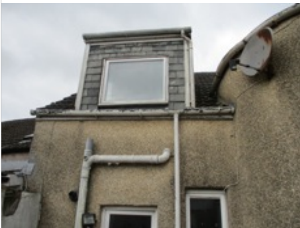
Rear Elevation - rainwater goods/soil and waste pipes - mixture of cast iron and pvc
