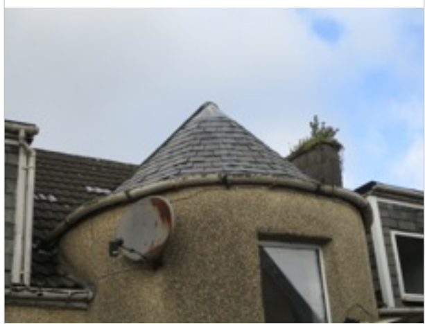
Rear Elevation - staircase projection - corrosion to cast iron gutters/uneven and loose/damaged fixings
