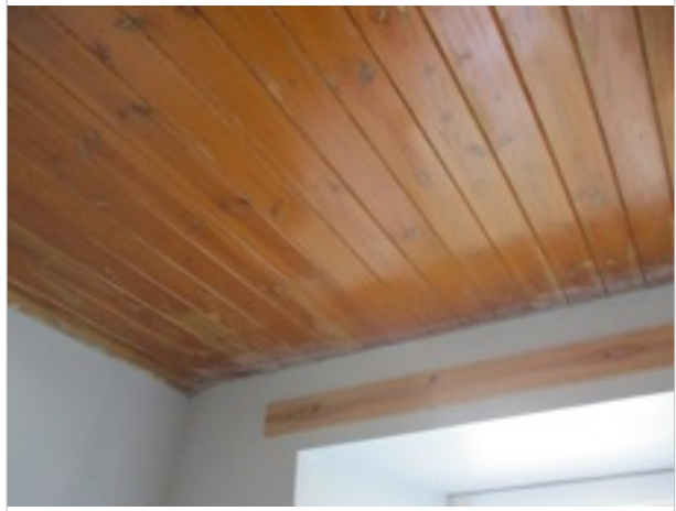
Living Room - some deterioration to varnish on timber clad ceiling
