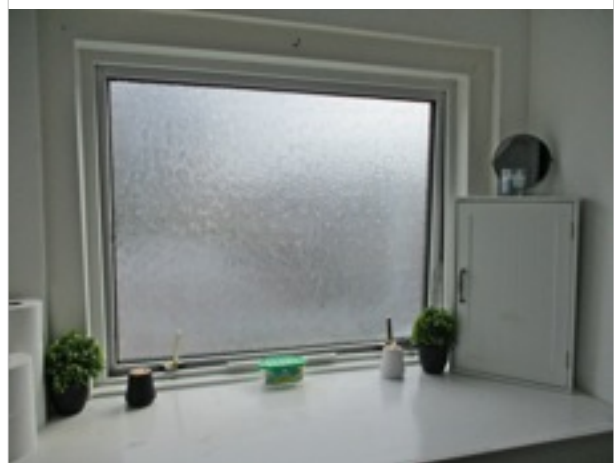
Bathroom - uPVC double glazed window - hard to close properly/possible defective hinges
