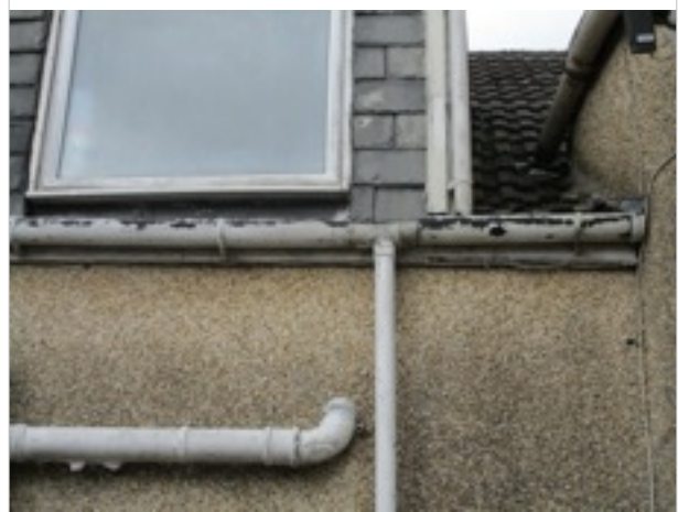
Rear Elevation - uneven/misaligned section of gutter at top of downpipe
