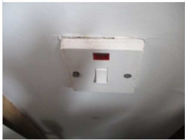
Living Room - switch for former electric storage heater - loose screws
