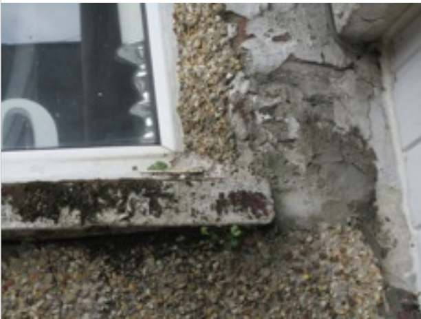
External view of Hall window showing extensive moss to concrete sill, vegetation growth and possible rot to timber above
