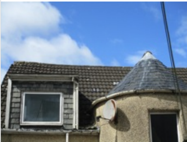
Rear Elevation - roof - sagging ridge line
