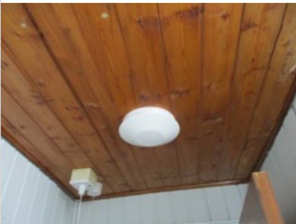
Bathroom - ceiling mounted extractor fan
