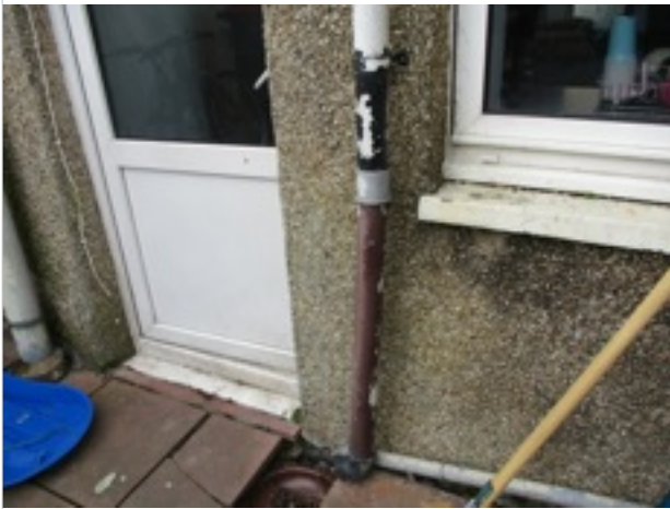
Rear Elevation - downpipe to right side of back door - sections mismatched/poor appearance
