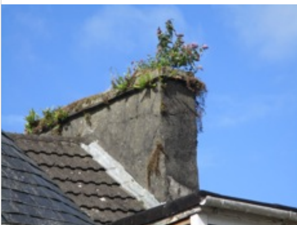
Rear Elevation - chimney - extensive vegetation growth
