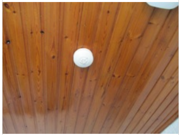
Kitchen - ceiling mounted heat detector (not working)
