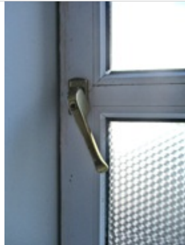
Living Room - window - not possible to open/ missing key/loose/damaged handle
