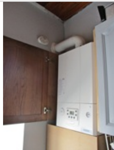
Kitchen - wall mounted CO detector (observation)
