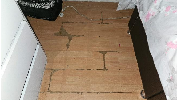
19 Example photograph of laminate flooring – Bedroom 2.
