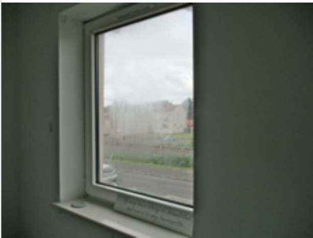
Front bedroom - left side window - double glazing seal failed causing build up of condensation between panes (observation)
