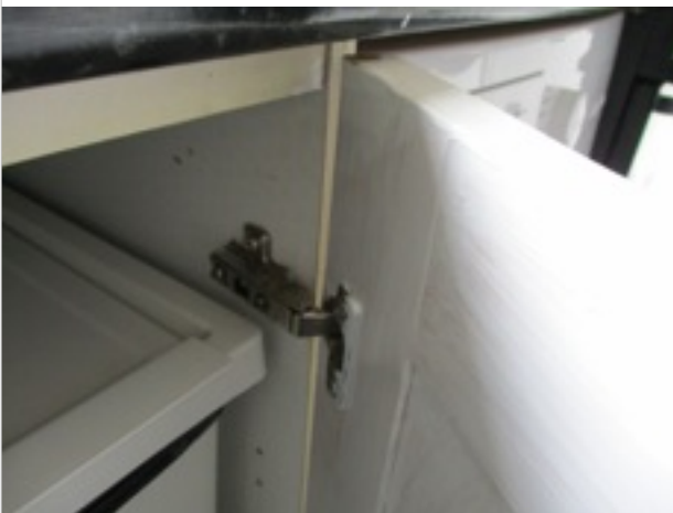
Kitchen - double base unit under sink - hinge to right side door loose/defective
