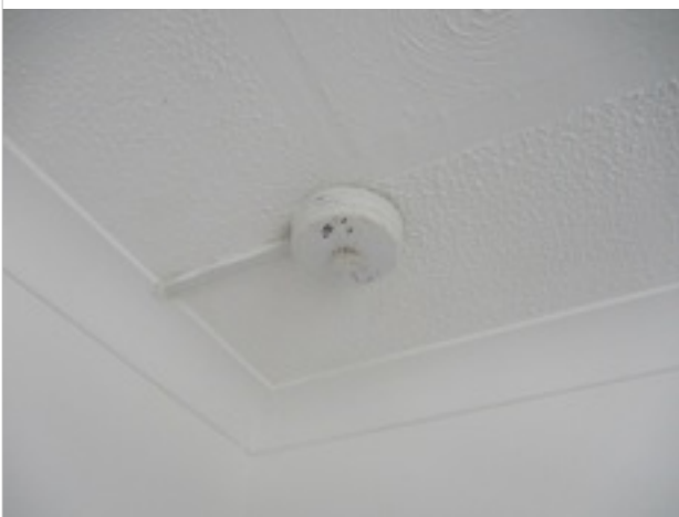
Kitchen - ceiling mounted heat detector (1) (observation)
