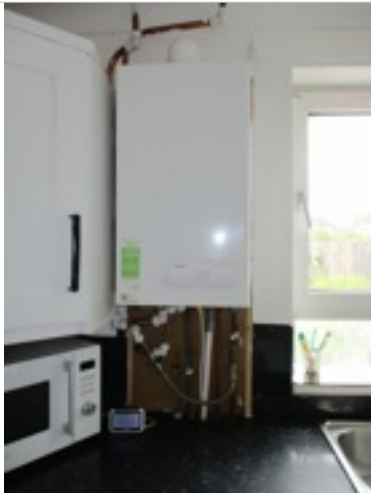
Kitchen - wall mounted boiler/exposed pipes
