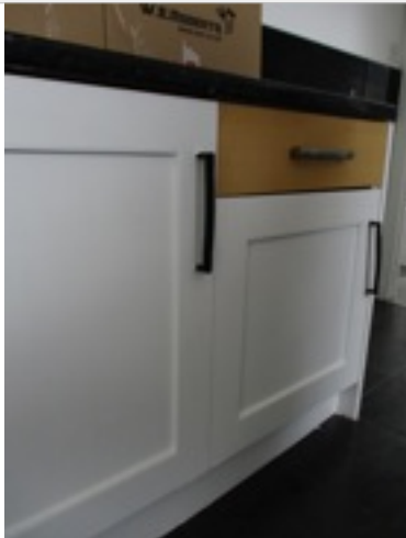
Kitchen - base units - mismatched/false drawer front fitted on end unit
