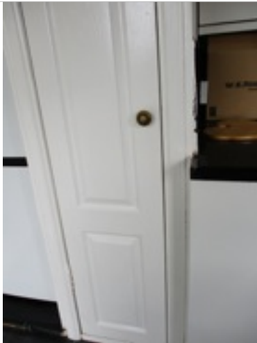
Kitchen - Large cupboard - door does not open and close properly/ill fitting and handle loose
