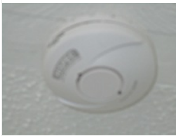
Kitchen - ceiling mounted heat detector (2) (observation)
