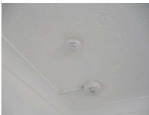
Living Room - 2 x ceiling mounted smoke detectors (observation)
