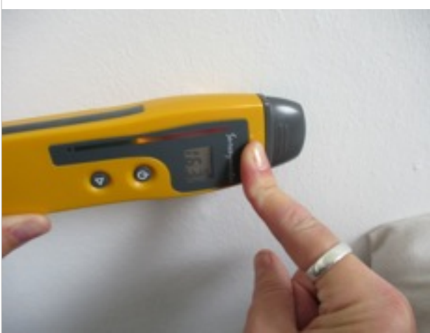
Front bedroom - internal party wall - damp meter reading showing moderate moisture level (search mode)
