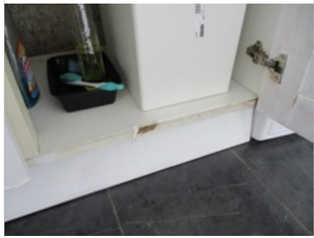
Kitchen - double base unit under sink - damage to base of unit on right side
