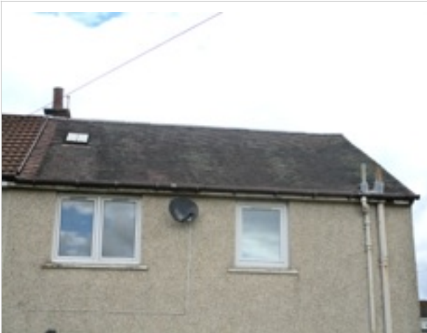
Roof - rear elevation - some deterioration to roof tiles
