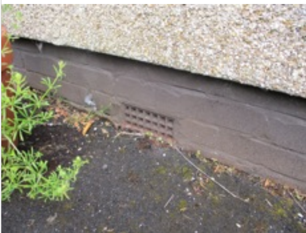
Gable wall - underfloor vent towards front - part covered by tarmac path surface
