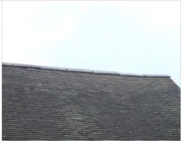
Roof - rear elevation - some deterioration to roof tiles/some tiles loose/dislodged/ridge tiles require re-bedding/pointing
