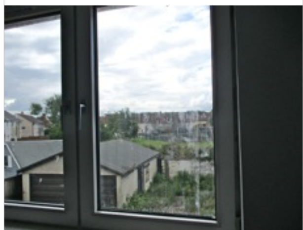
Rear bedroom (1) - window - double glazing seal to right side failed causing build up of condensation between panes (observation)
