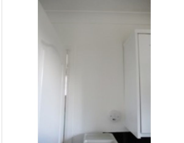
Kitchen - wall mounted carbon monoxide detector (observation)
