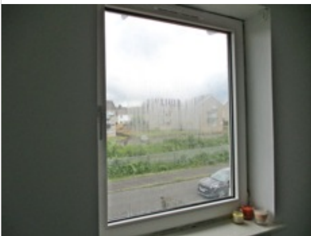
Landing - window - double glazing seal failed causing build up of condensation between panes (observation)
