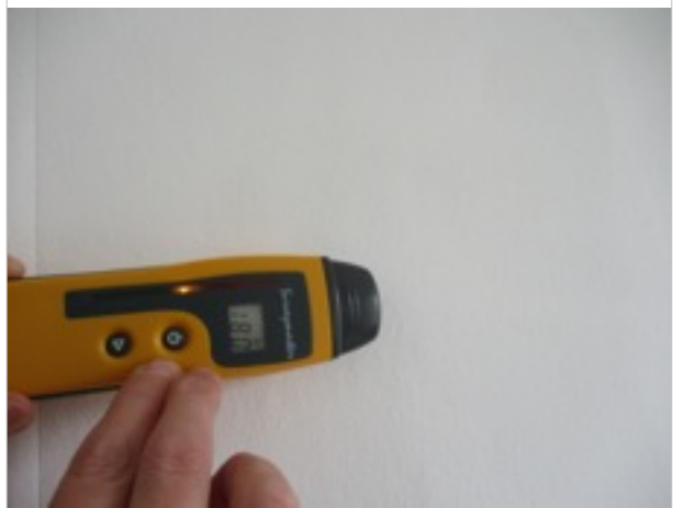
Front bedroom - internal party wall - damp meter reading showing moderate moisture level (search mode)
