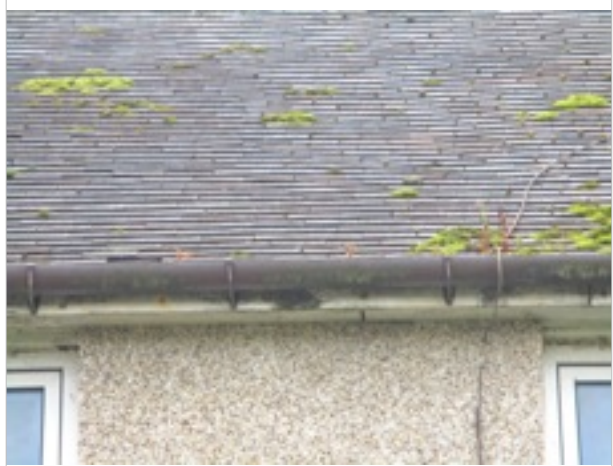
Roof - front elevation - some dislodged roof tiles/patches of moss/build up of vegetation in gutter
