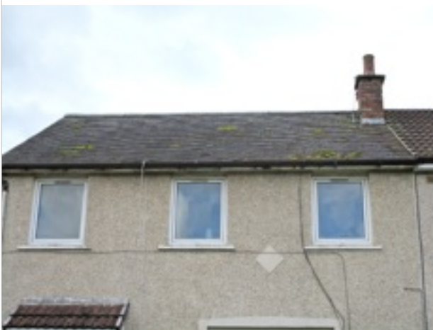
Roof - front elevation - some deterioration to roof tiles
