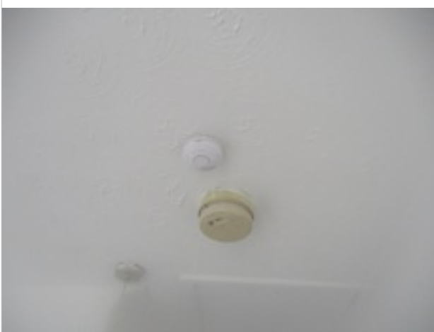
Landing - 2 x ceiling mounted smoke detectors (observation)
