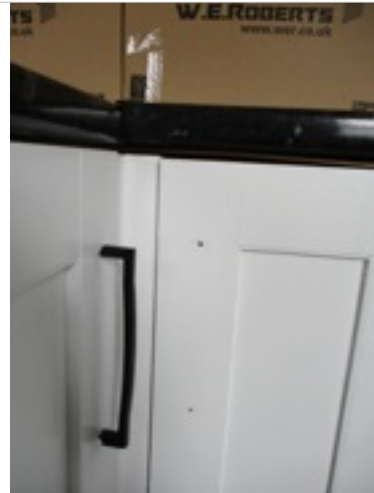
Kitchen - corner base unit - doors do not open and close properly/misaligned/loose/defective fittings and missing door handle
