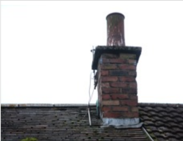
Roof - front elevation - chimney requires pointing/possible loose flashings
