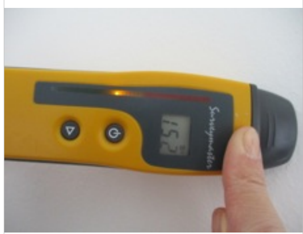
Front bedroom - front elevation between windows - damp meter showing moderate moisture level (search mode)
