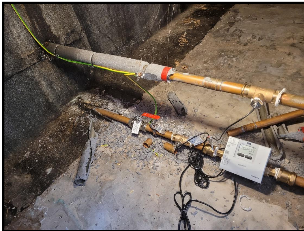
Photograph 5 Sun lounge underfloor – Recently fitted heat meter.
