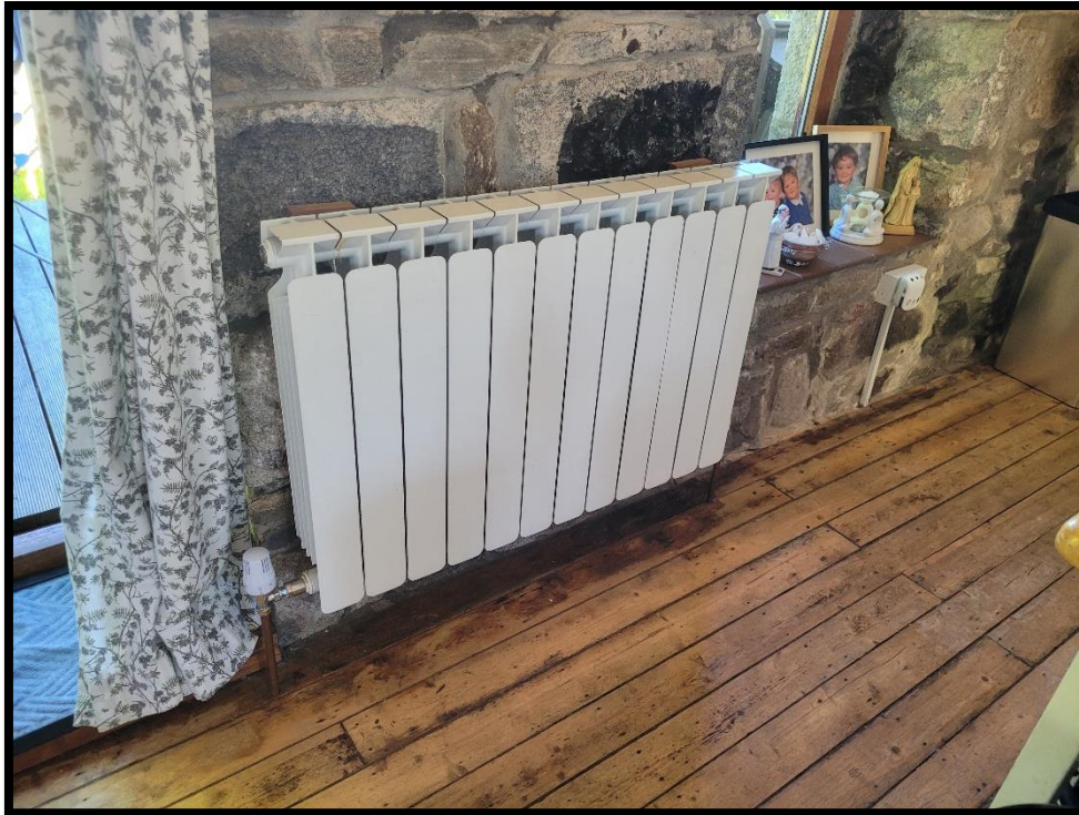
Photograph 2 Kitchen – typical radiator with thermostatic valve
