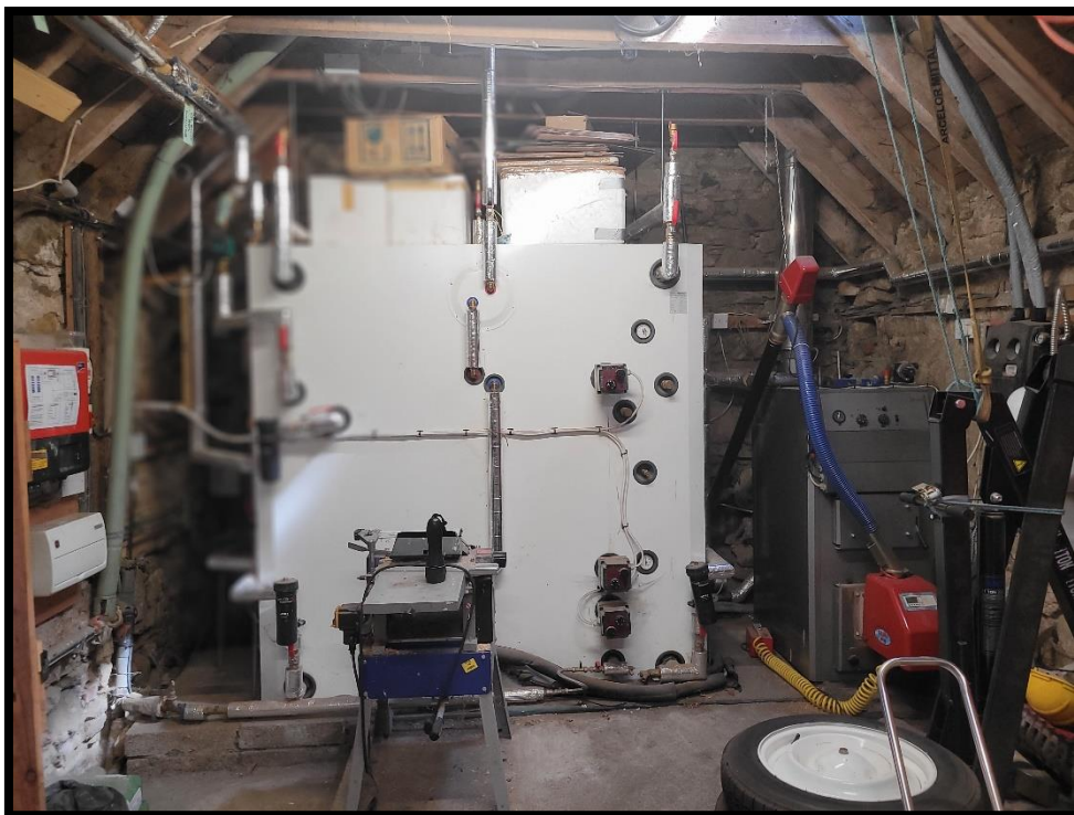
Photograph 6 Outbuilding – Communal central heating boiler and accumulator tank.
