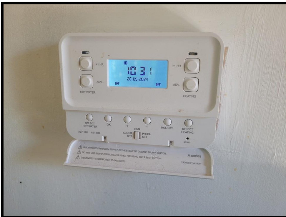
Photograph 3 Kitchen – Central heating and hot water programmer.
