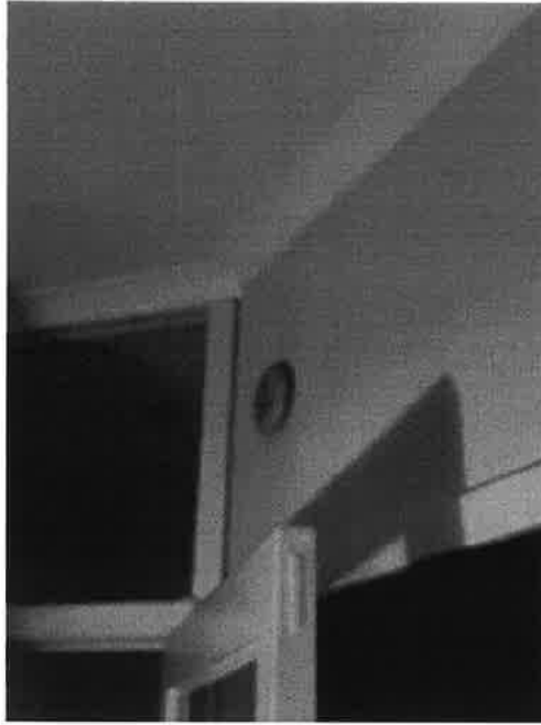
Photograph 6: Hallway: smoke detector
