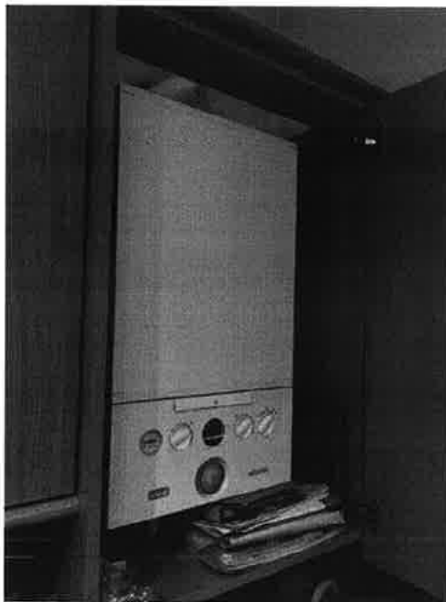
Photograph 5: Kitchen gas boiler
