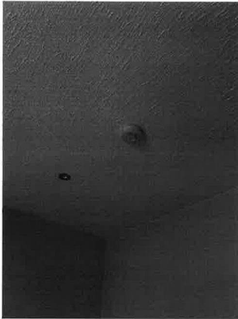
Photograph 2: Kitchen: heat detector
