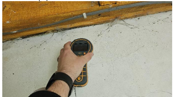
20 High qualitative moisture readings to separating wall between "coal bunker" and kitchen.
