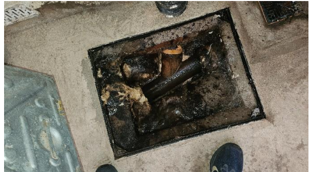
18 Inspection chamber to underground drainage – note: toilet paper debris.
