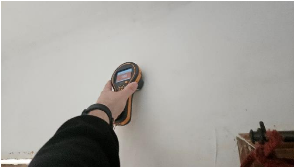
11 Elevated qualitative moisture meter readings above "coal bunker" door.
