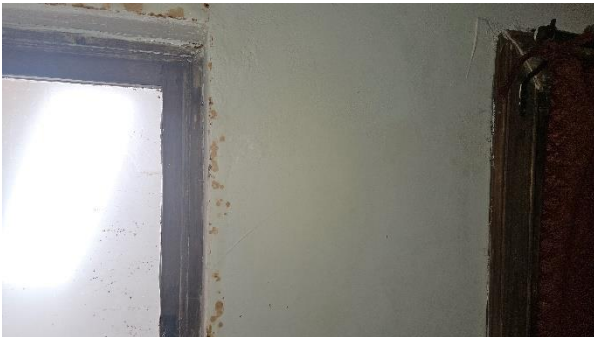
5 View of visual staining around Kitchen window.
