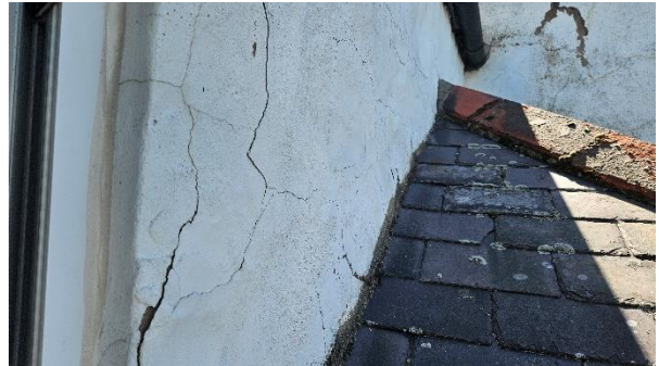
26 Poor condition of render to rear elevation at first floor level and poor skew detail to junction with slatework.
