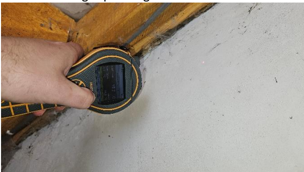
21 Condensation assessment – "coal bunker" walls 1.7°C above dewpoint at time of inspection.
