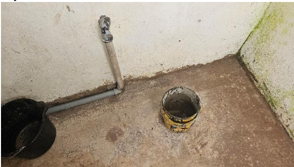
15 Kitchen sink waste, buckets set on floor.
