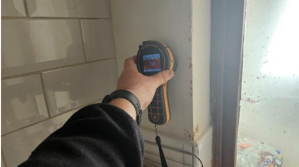
13 Elevated qualitative moisture meter readings adjacent to kitchen window.
