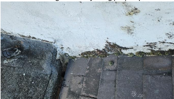
29 Poor skew detailing extending into gutter and over stop end, presence of moss growth at cracks indicating moisture retention.
