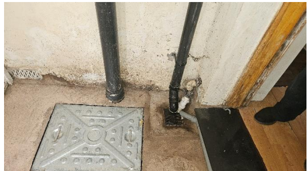
16 Soil and drainage pipework within "coal bunker".
