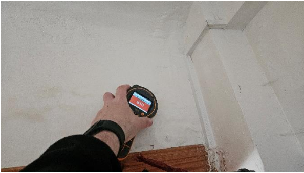
9 Elevated qualitative moisture meter readings above "coal bunker" door.
