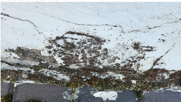
31 Poor skew detailing, presence of moss growth at cracks indicating moisture retention.
