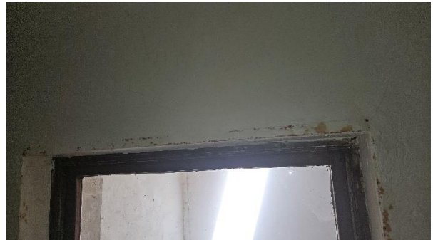
6 View of visual staining around Kitchen window.
