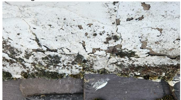
30 Poor skew detailing, presence of moss growth at cracks indicating moisture retention.
