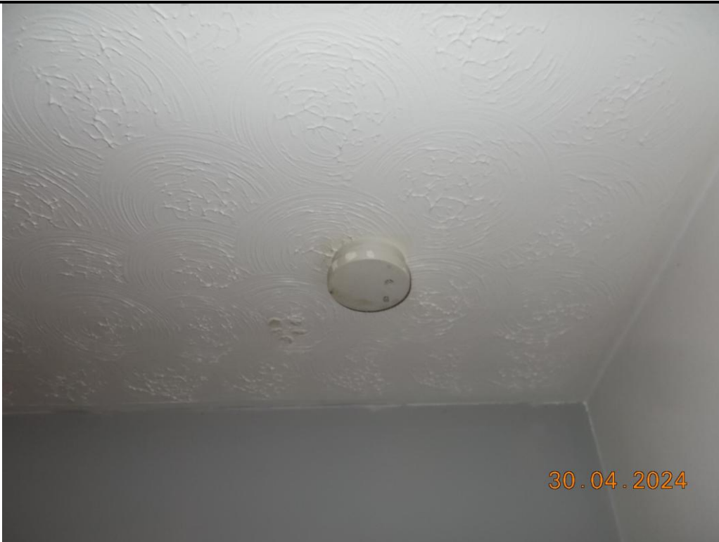
4. Smoke Alarm in Bed sitting Room
