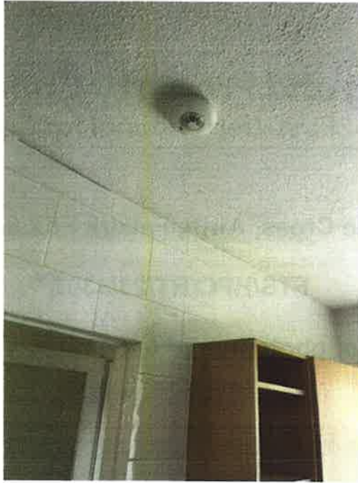
Photograph 2: Kitchen: heat detector
