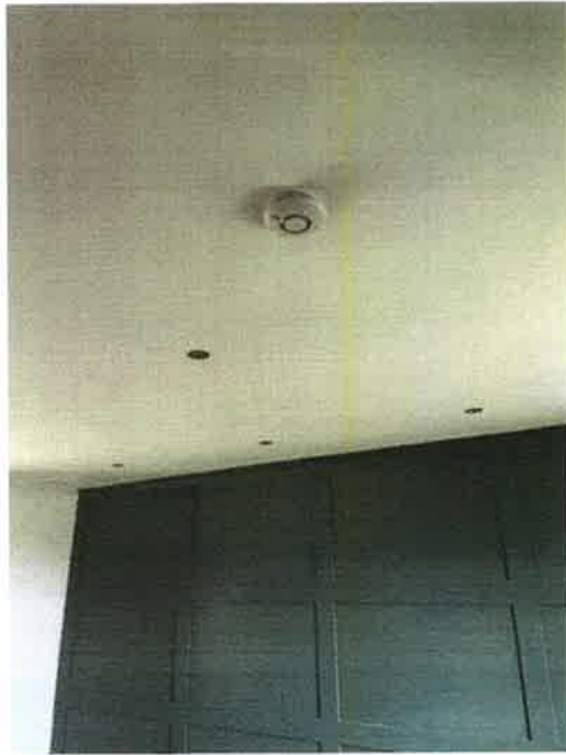
Photograph 4: Living room: smoke detector
