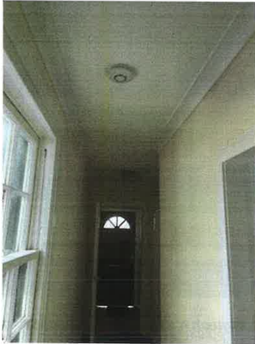
Photograph 6: Hallway: smoke detector
