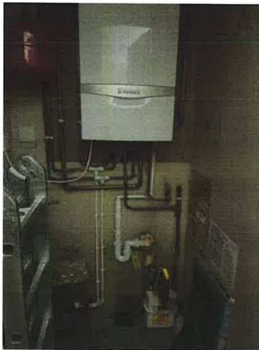
Photograph 7: Gas boiler in Elphinstone Inn (adjacent): said to feed into boiler at subject showing pipe cut on right hand side
