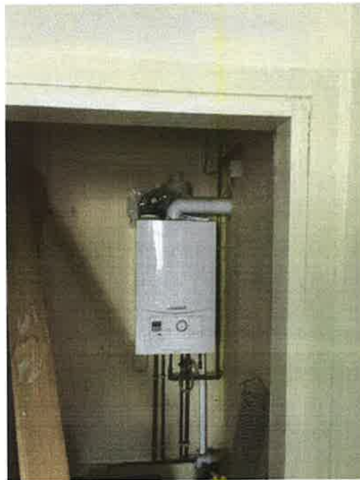
Photograph 5: Living room: gas boiler – said to be disconnected; no carbon monoxide detector
