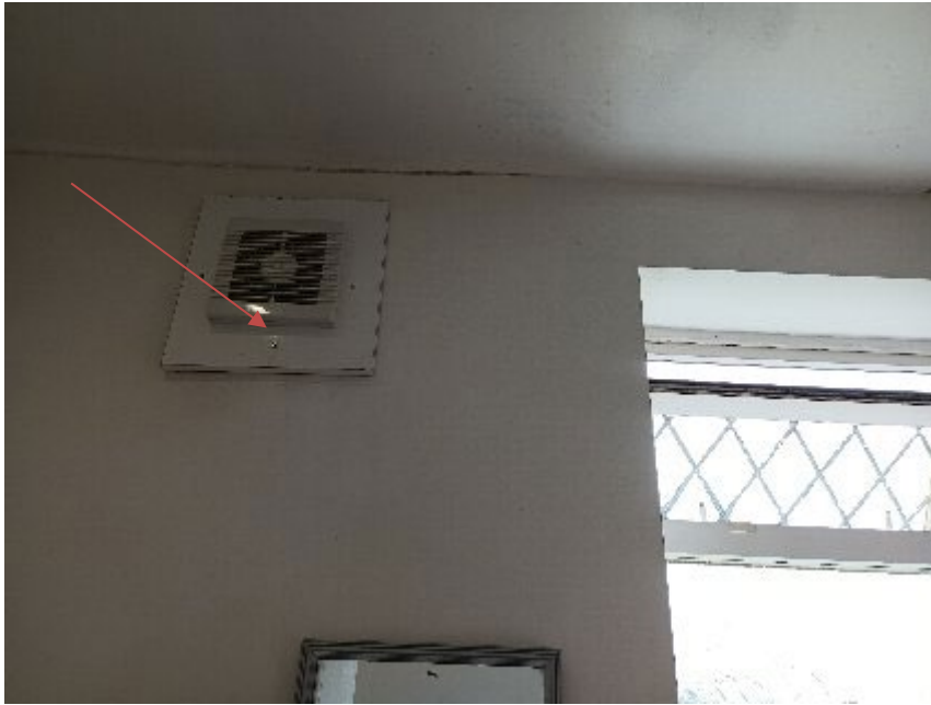
8 Recently installed fan in bathroom
