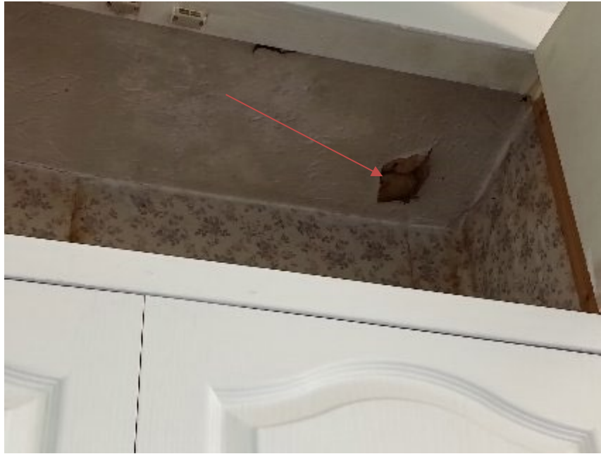
4 Damaged plaster in the cupboard middle west room
