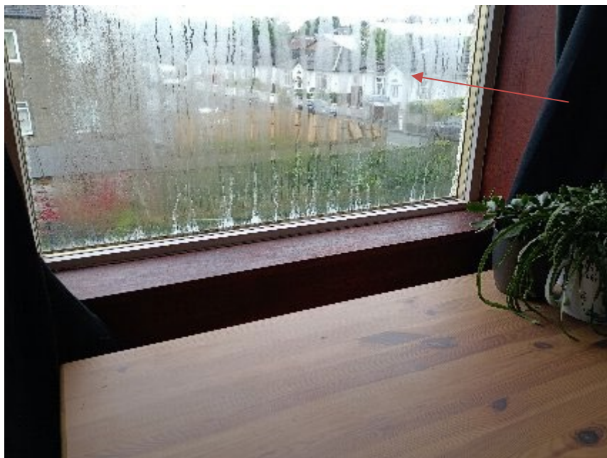
5 Defective glazing panel seals in rear north room
