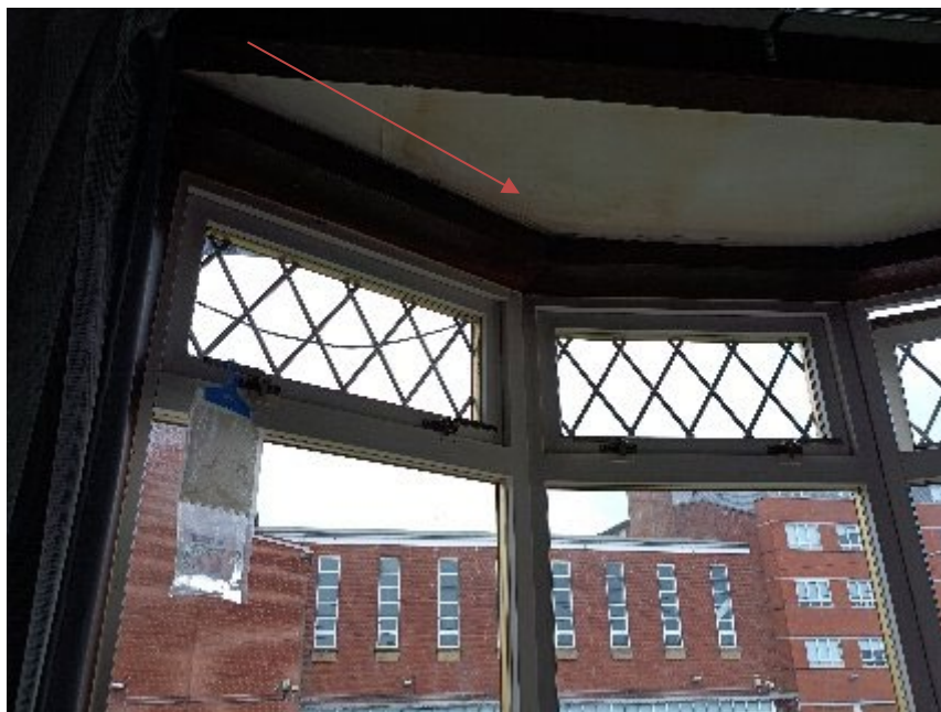
7 Residual staining at east lounge ceiling
