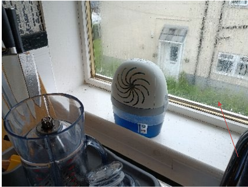
6 Defective glazing panel seals in kitchen
