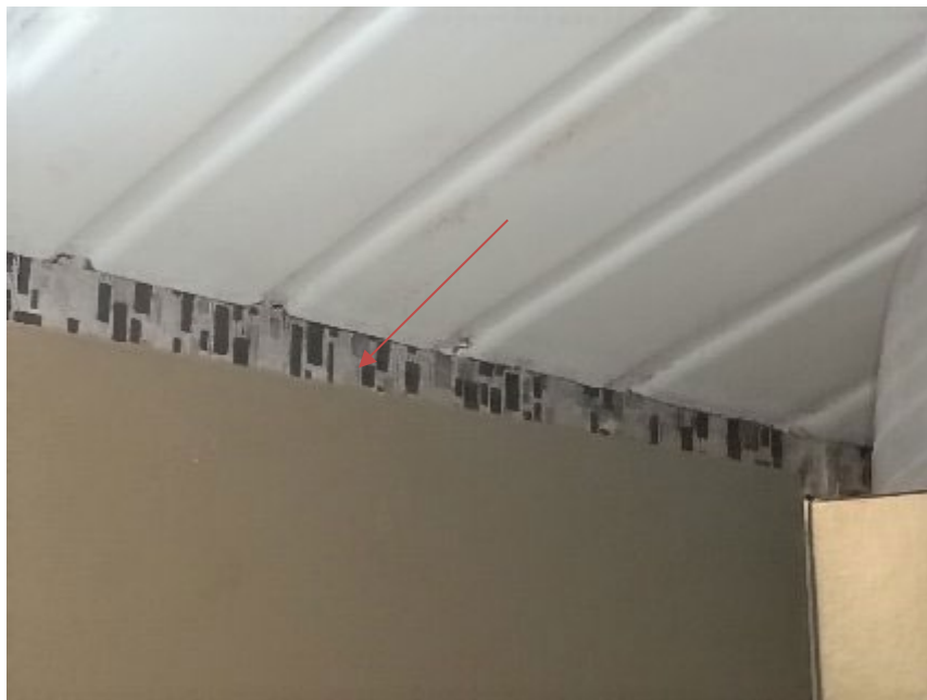
3 Residual damp staining ceiling level west in the kitchen
