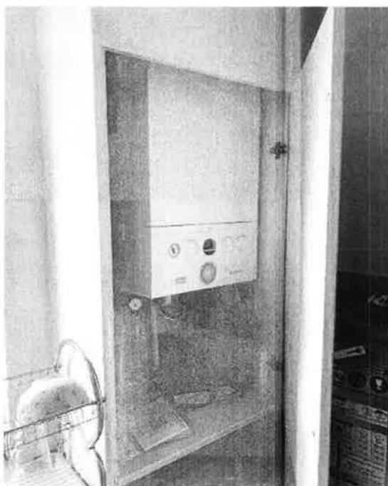
2. Wall mounted boiler in kitchen
