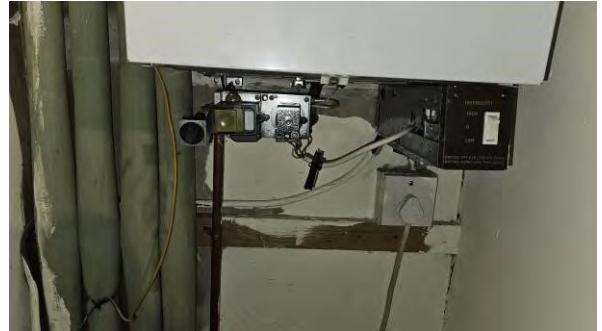
2 Gas fired boiler not operational.
