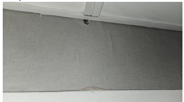
14 Minor adjacent above Kitchen door at cable penetration from smoke/heat detector cabling.
