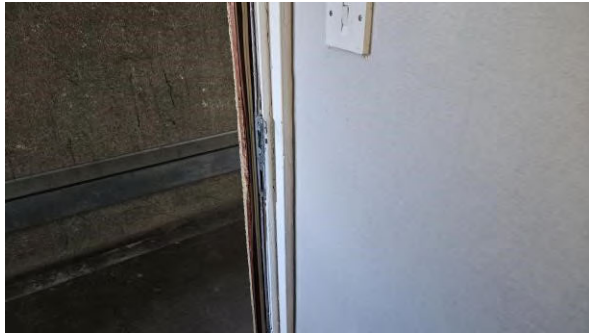
9 Front door – defective door stop.
