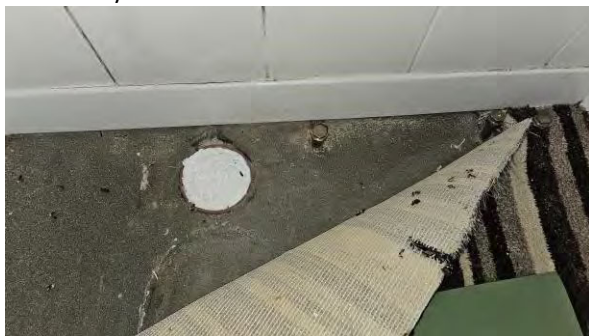
13 Poor silicon sealant capping to soil pipe.
