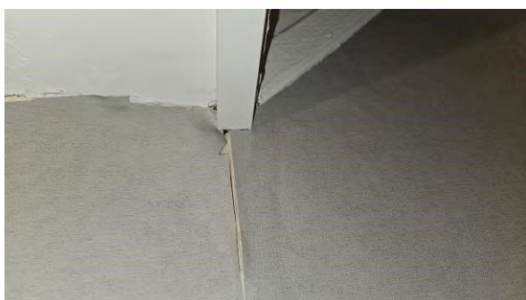
15 Minor damage at circulation corridor adjacent to cabling penetration.
