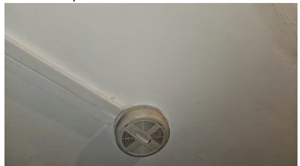
6 Satisfactory smoke detection.
