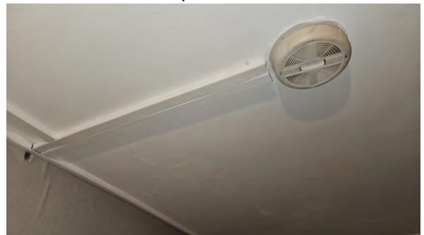
4 Satisfactory smoke detection.
