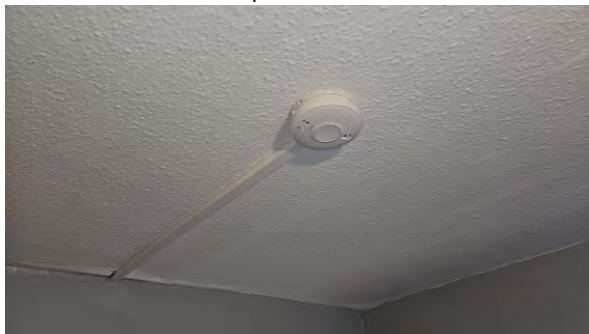
3 Satisfactory smoke detection.
