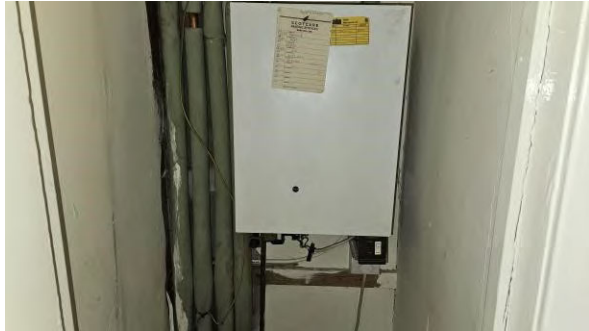
1 Gas fired boiler not operational.
