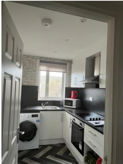
Photograph 3: Kitchen ceiling (with heat detector)
