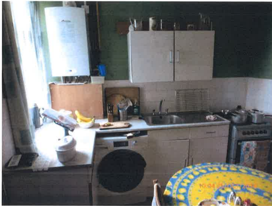
Kitchen showing the central heating boiler
