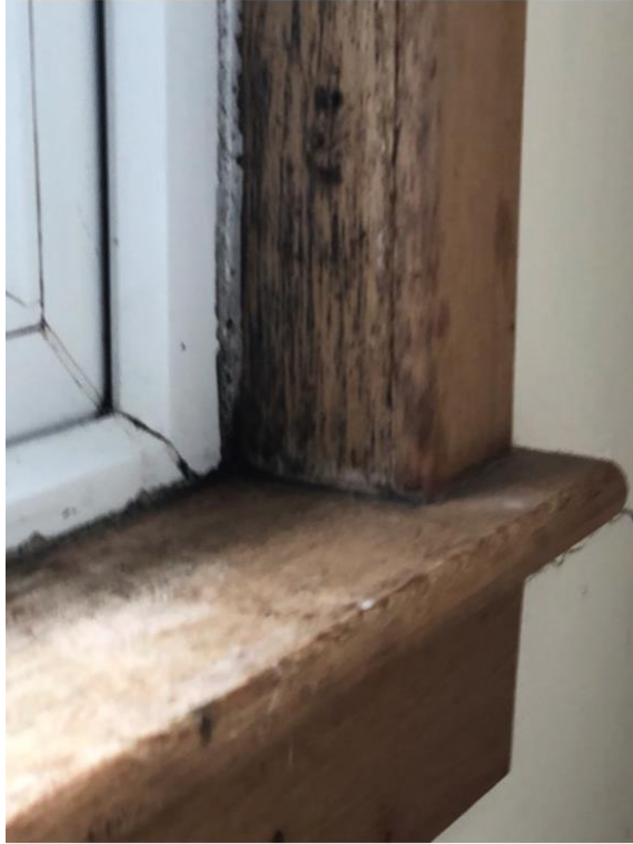
Photo 6 – Water damage to upper-right bedroom sill
