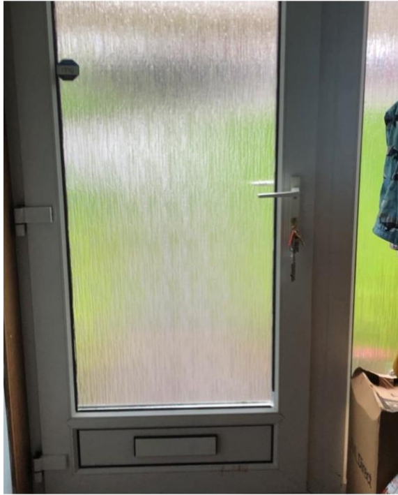
Photo 2 – Correctly functioning front door and lock
