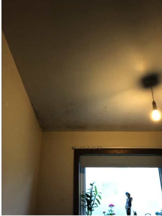
Photo 18 – Mould on G/F Bedroom ceiling
