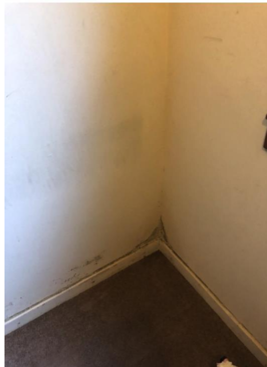
Photo 17 – Dampness and mould in G/F bed.
