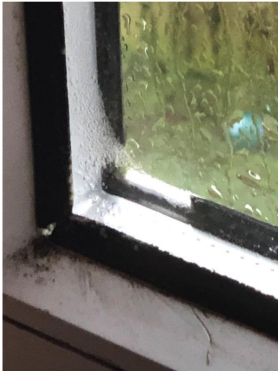
Photo 12 – Window seals incomplete/damaged
