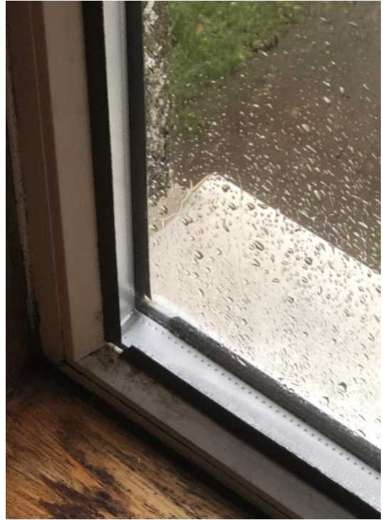
Photo 11 – Window seals incomplete/damaged
