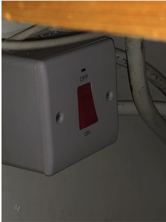
Photo 14 – Replacement shower switch near boiler
