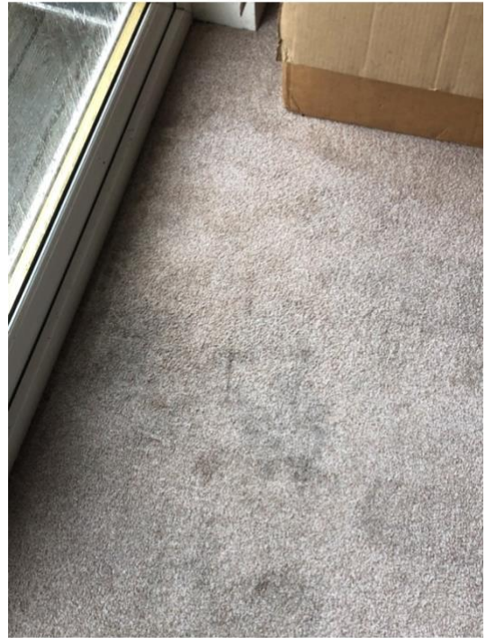
Photo 3 – Saturated carpet at patio door
