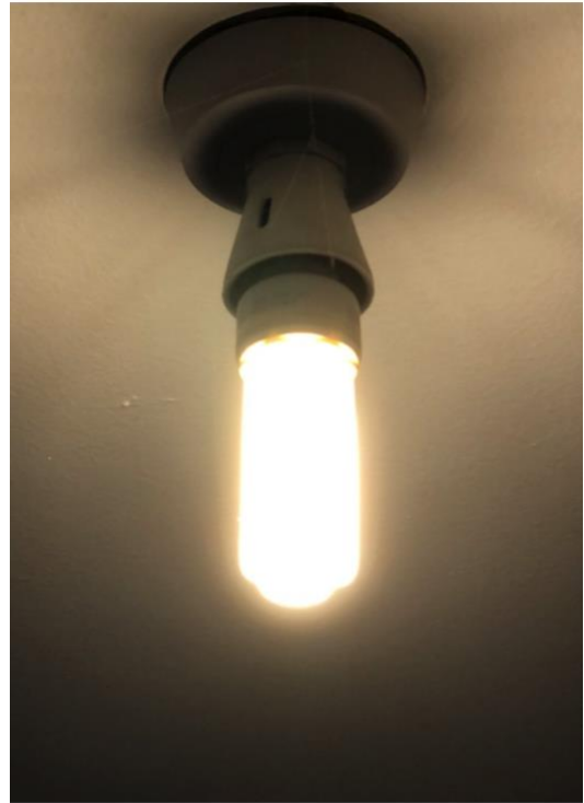
Photo 15 – Inappropriate bathroom light fitting
