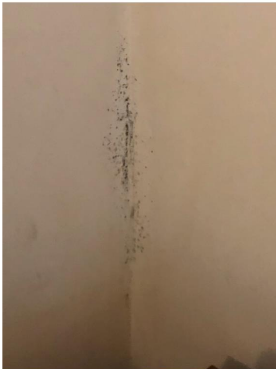
Photo 4 – Surface mould on living room wall
