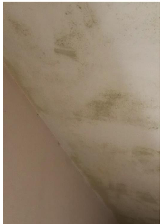
Photo 9 – Mould on upper-left bedroom ceiling
