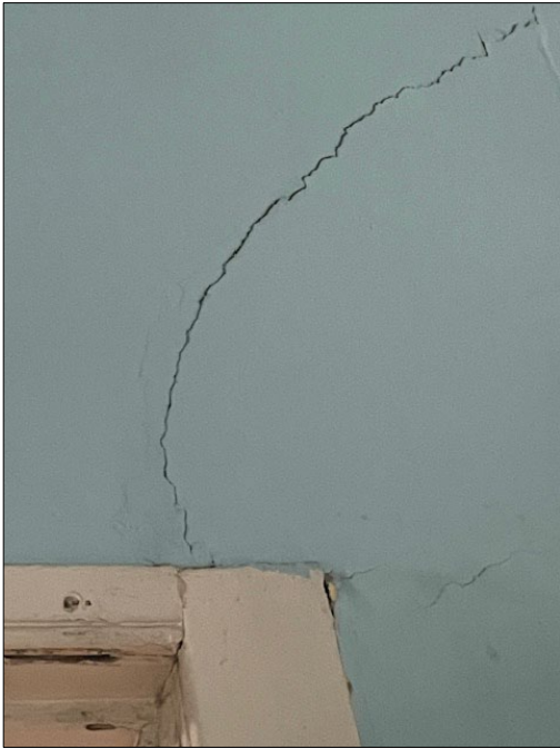
Cracking in kitchen above door to hall.
